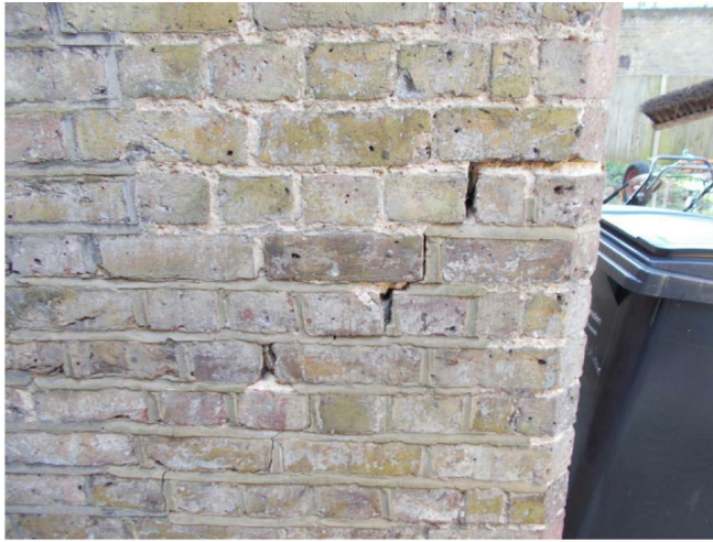
View of damage to rear right corner
