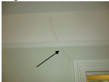
Cracking in Flat C lounge
