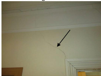
Cracking in Flat B rear left hand bedroom
