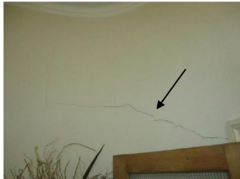
Cracking in Flat A hall
