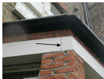
Cracking to rear bay
