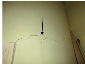
Cracking in Flat A kitchen
