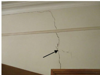
Cracking in Flat A lounge
