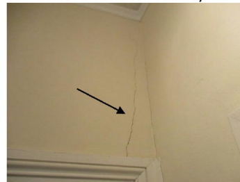
Cracking in Flat B hall
