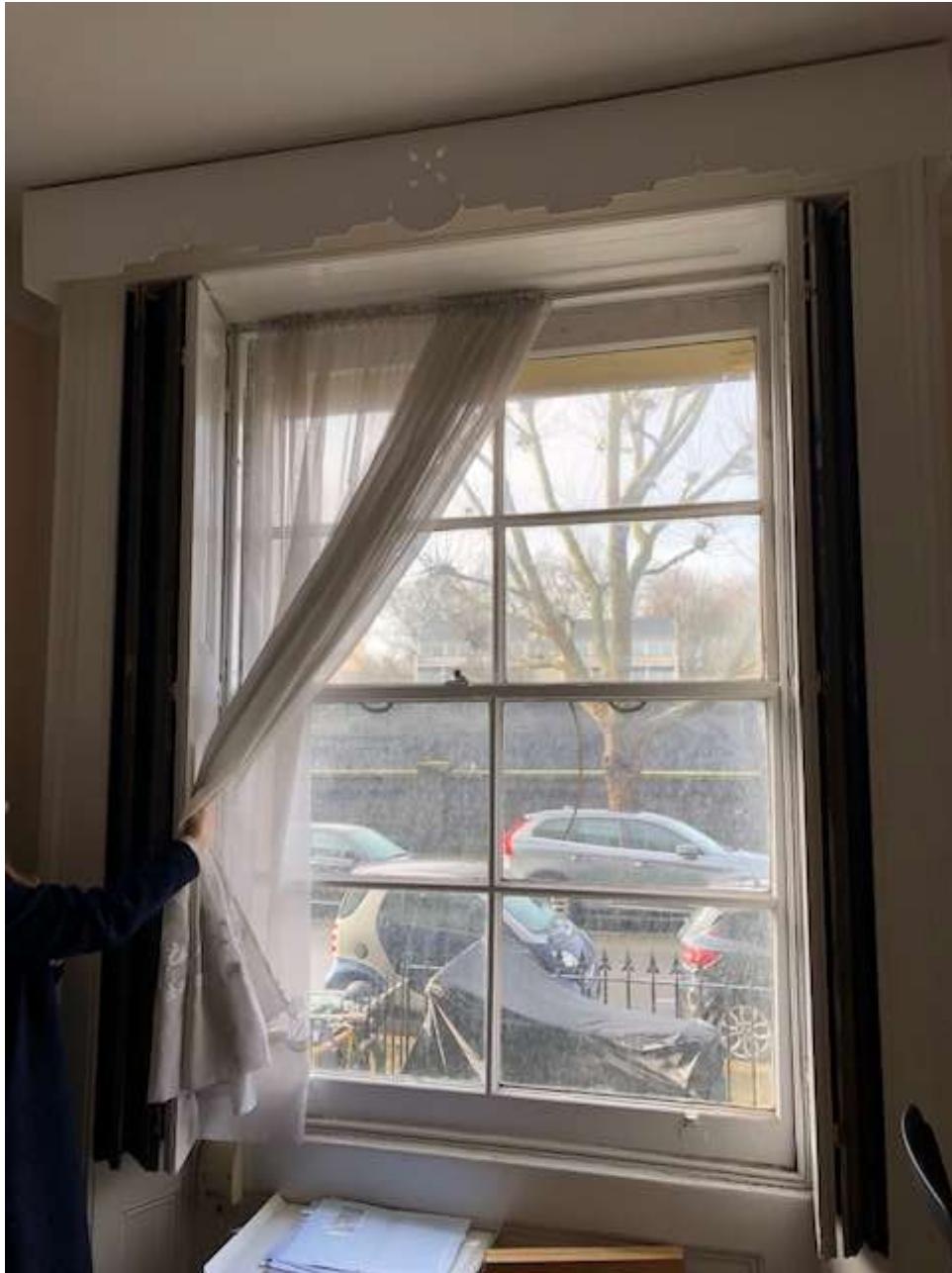
Figure 5: Internal view of the window in the living room at ground floor
