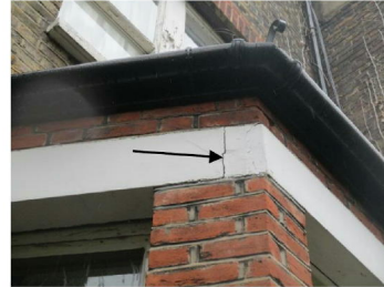
Cracking to rear bay
