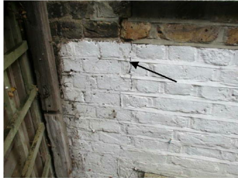
Cracking to rear elevation
