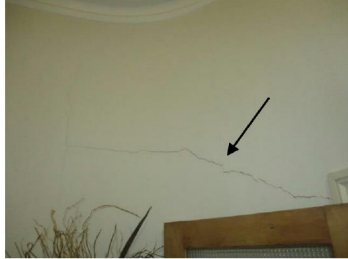
Cracking in Flat A hall
