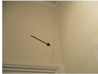
Cracking in Flat B hall
