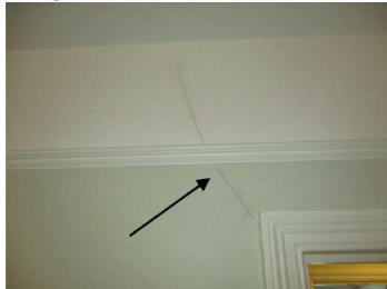
Cracking in Flat C lounge
