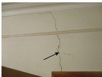
Cracking in Flat A lounge
