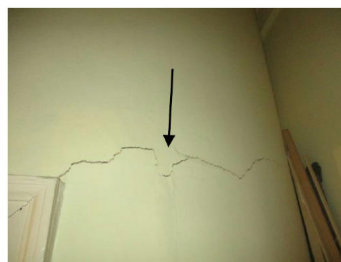
Cracking in Flat A kitchen
