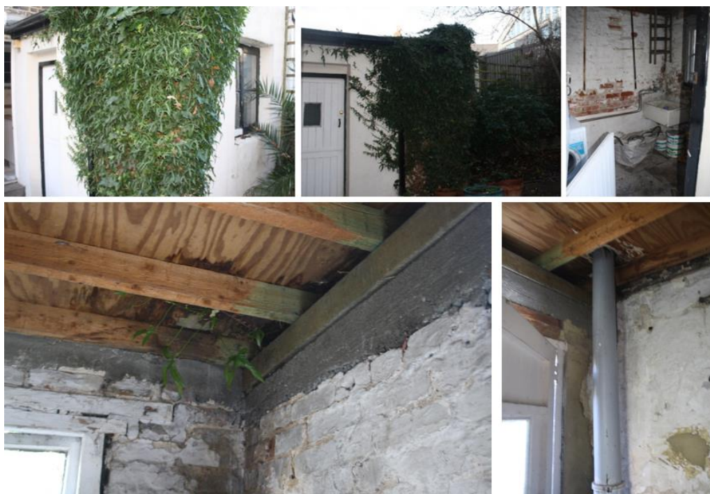
POOR QUALITY OF EXISTING REAR EXTENSION
