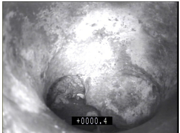
Photo: 5_5a 0.4m, Collapsed Pipe, 95 % cross-sectional area loss
