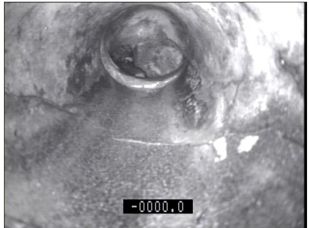
Photo: 3_3a 0m, Circumferential Crack, from 03 to 08 o'clock
