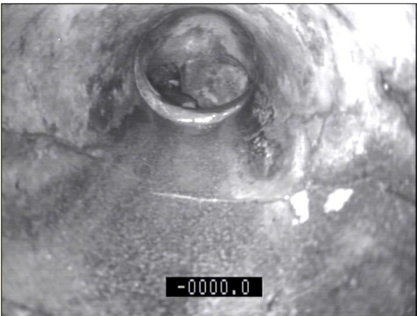
Photo: 4_4a 0m, Line of Sewer deviates up
