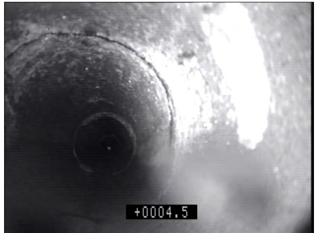
Photo: 18_7a 4.5m, Circumferential Crack, from 10 to 02 o'clock
