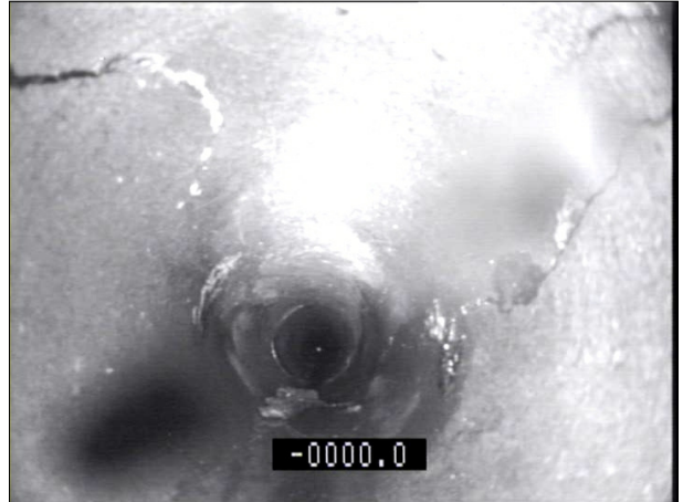
Photo: 14_3a 0m, Longitudinal Fracture at 10 o'clock
