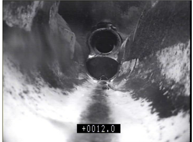
Photo: 22_11a 12m, Manhole Remark: IC1/INT
