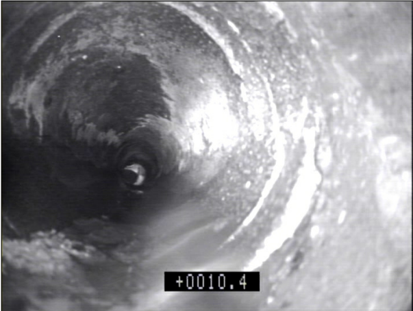
Photo: 21_10a 10.4m, Circumferential Fracture, from 03 to 09 o'clock
