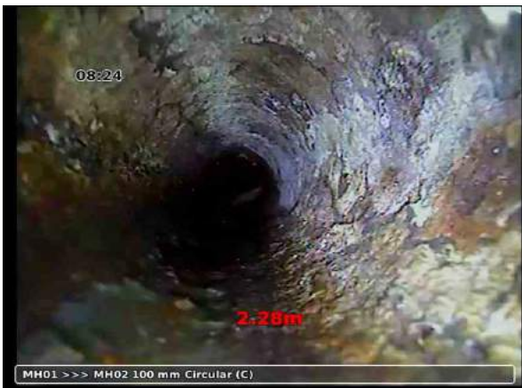
, 00:00:45, 2.28 m Settled deposits, fine, 5% cross-sectional area loss
