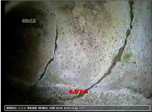
, 00:00:55, 4.07 m Fracture, circumferential from 1 o'clock to 5 o'clock
