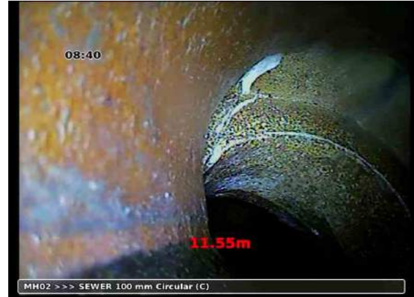
, 00:01:54, 11.55 m Broken pipe from 10 o'clock to 1 o'clock
