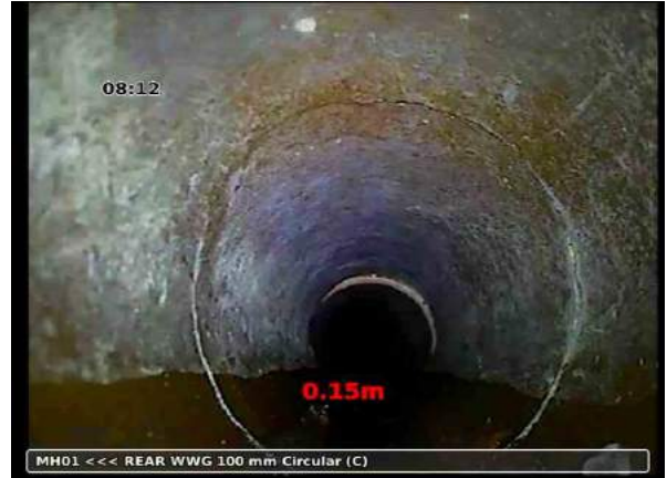
, 00:00:22, 0.15 m Fracture, circumferential from 12 o'clock to 12 o'clock
