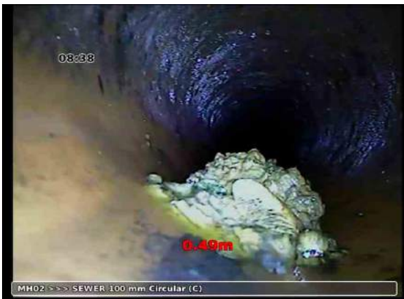
, 00:00:18, 0.49 m Settled deposits, coarse, 15% cross-sectional area loss
