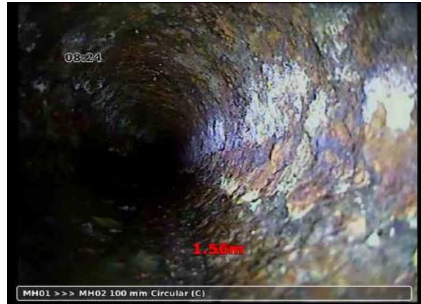
, 00:00:39, 1.60 m Settled deposits, fine, 10% cross-sectional area loss
