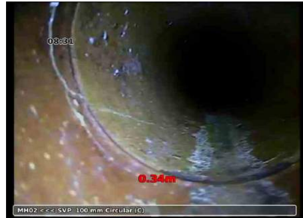
, 00:00:25, 0.34 m Crack, circumferential from 7 o'clock to 11 o'clock
