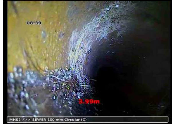
, 00:00:58, 3.99 m Roots, mass at joint, 5% cross-sectional area loss
