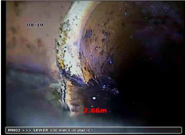
, 00:00:46, 2.66 m Pipe material changes to vitrified clay at this point
