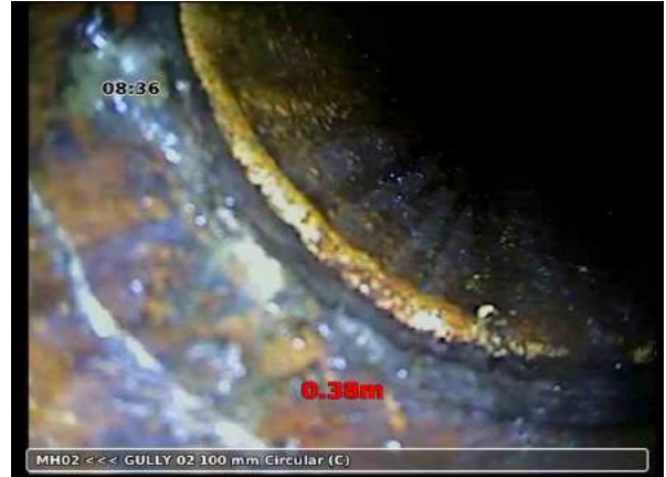
, 00:00:17, 0.38 m Fracture, circumferential from 6 o'clock to 8 o'clock
