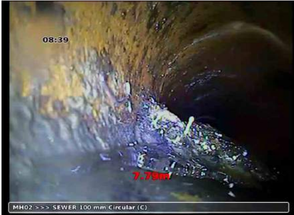
, 00:01:26, 7.79 m Attached deposits, encrustation from 5 o'clock to 8 o'clock, 20% cross-sectional area loss
