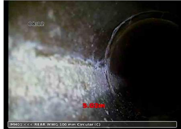
, 00:01:00, 5.02 m Fracture, circumferential from 8 o'clock to 2 o'clock
