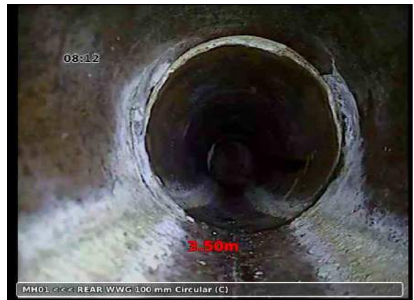
, 00:00:49, 3.50 m Crack, circumferential from 7 o'clock to 11 o'clock
