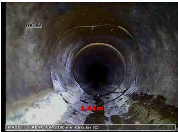
, 00:00:33, 1.41 m Fracture, circumferential from 12 o'clock to 12 o'clock
