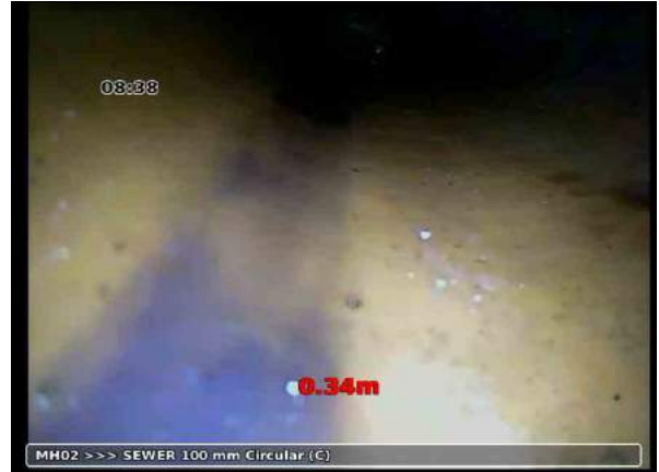
, 00:00:17, 0.19 m Pipe material changes to polyvinyl chloride at this point
