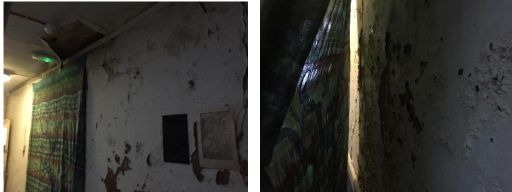
Figures 2 and 3: Water damage to interior wall of the hallway at the second floor level (Source: Icen Projects Ltd, Site visit conducted on 8 March 2017)
