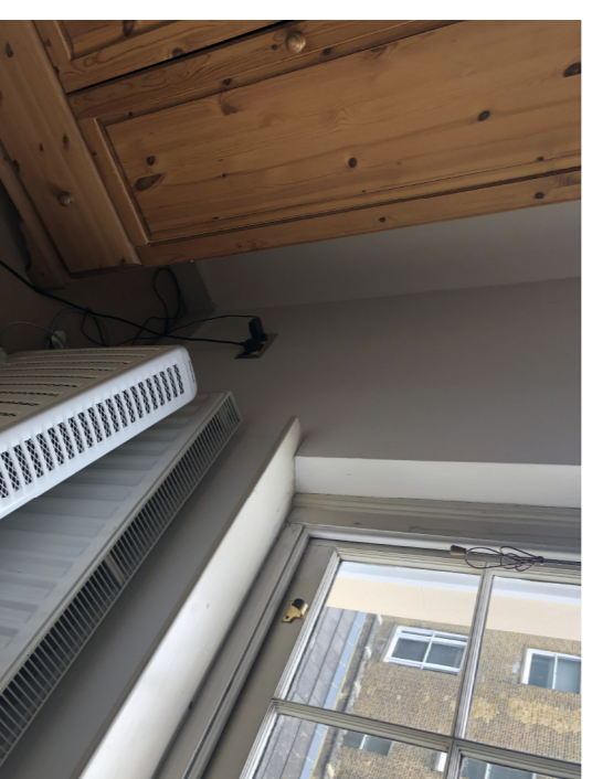
SLIGHT CRACKING ABOVE AND BELOW WINDOW REPAIR A PHOTO 52
