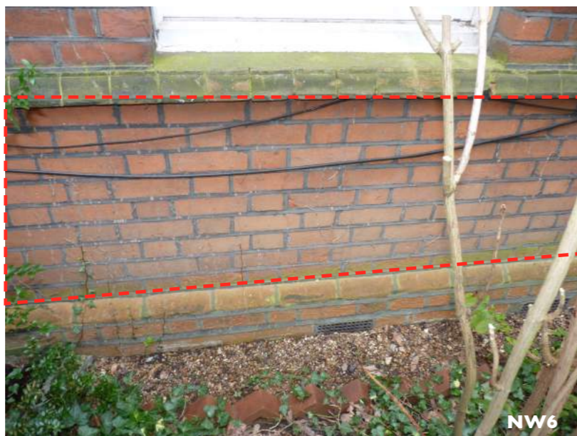
Photos NW5-NW6 Red dashed line denotes the repointing work that was carried out to the ground floor walls. Some of the windows were drought proofed with caulk which is visible on photo NW7
