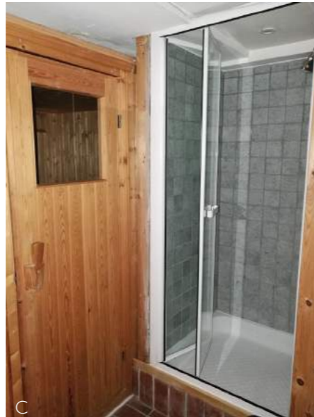
Photos A-C Photo A shows the staircase. Photo B shows new pier column which supports new beam. Photo C shows timber partition between the sauna and shower.
