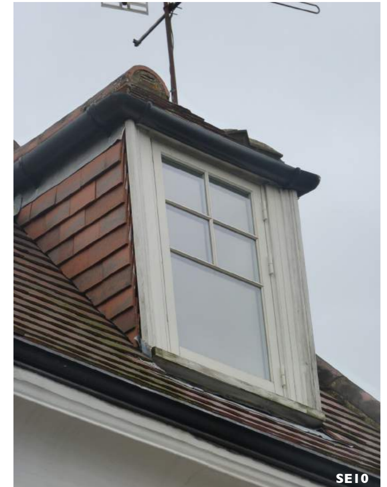
Photos SE9-SE10 Existing second floor dormer windows on South -East Elevation. These are modern timber casement windows.
