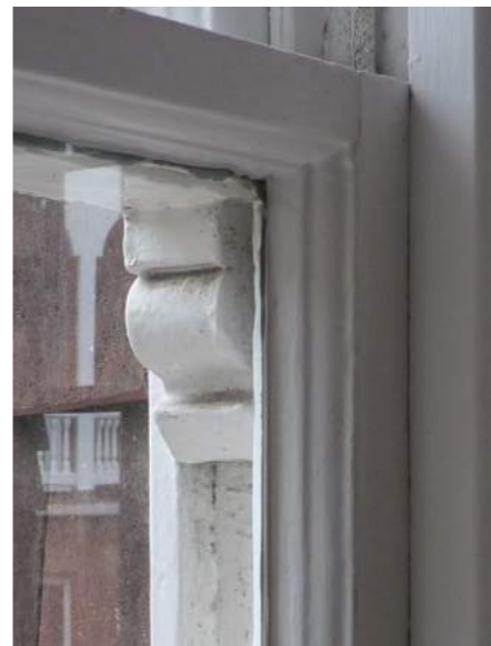
The horn detail shown is typical of the sashes to the ground floor and would appear to be original.
