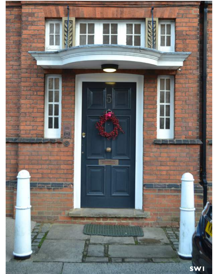
Photo SW1 Existing main entrance on South -West Elevation. The door is relatively modern however the side windows and the fan windows above canopy appear to be original.
