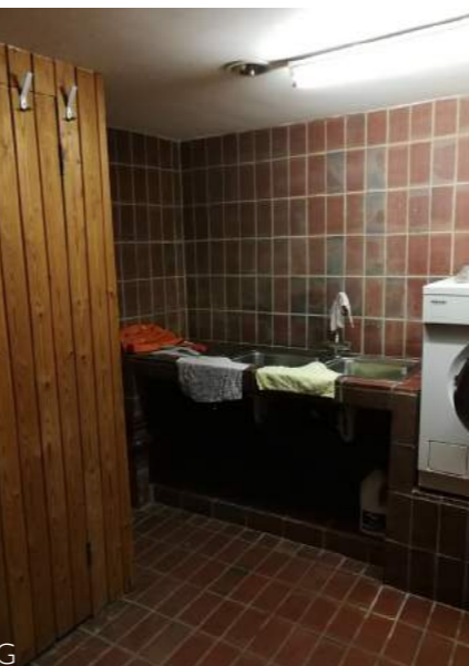
Photos D-G These photos show boxing in to the original lightwell windows as well as the remains of an original arch to the kitchen hearth which now holds new boiler. Photo G shows utility area to the back of the basement.
