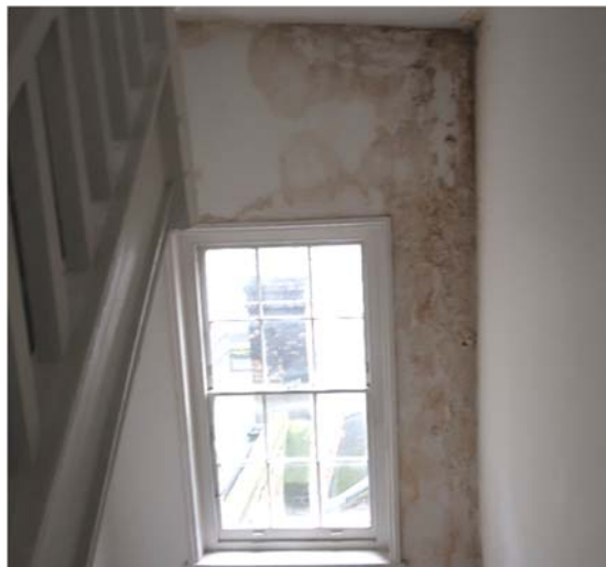
Leak from the Third Floor on the Second Floor stairwell
