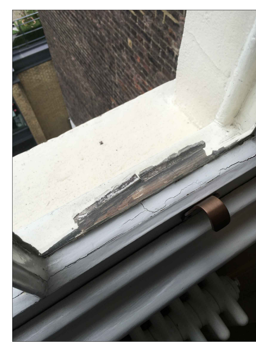
PHOTOGRAPH OF DAMAGED LOWER SASH WINDOW
