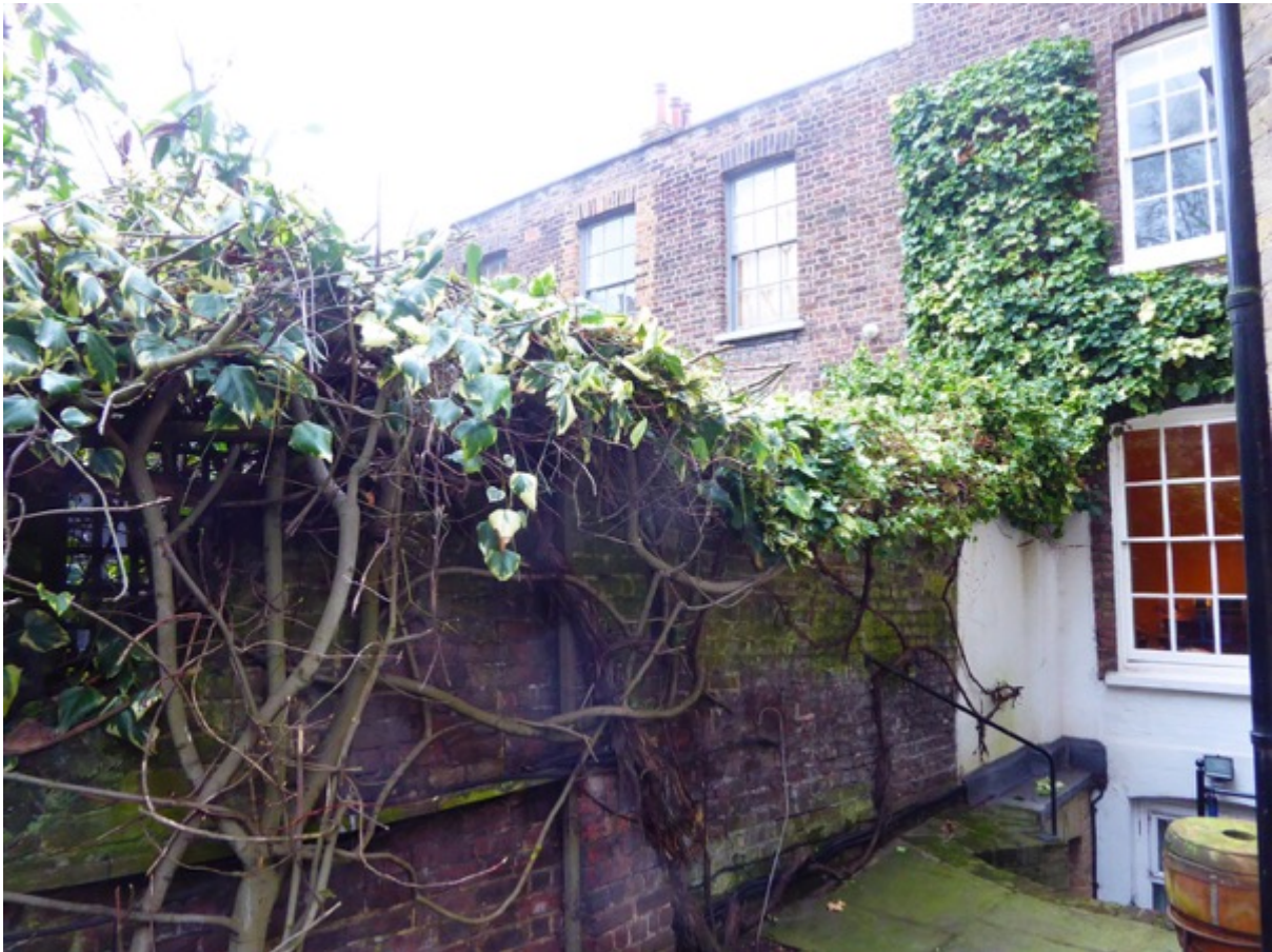
5. View of the boundary between No 7 and No 9. The proposed extension would rise 550mm above the top of the wall.
