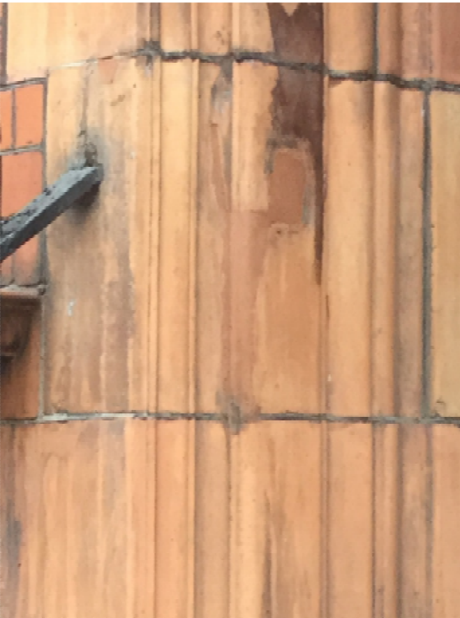
8. Shows close up of area where the original gates have been removed from Flat 60. Terracotta made good, as per proposal.
