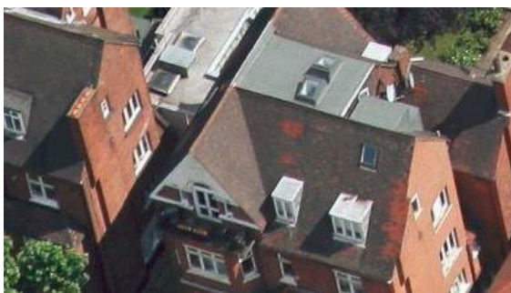
Pic. 8 - no. 10 unlawful rooflight
