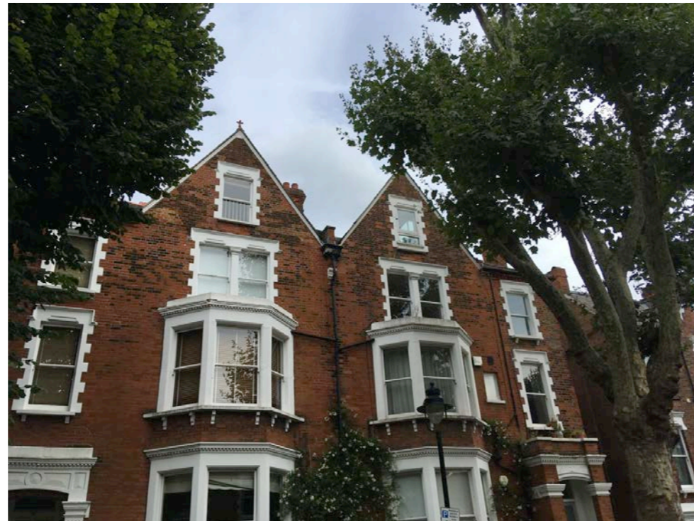
19 Tanza Road (Left) showing timber sash window in front gable. 17 Tanza Road (Right) has centre pivot window with fixed panel below. To be replaced with timber sash window to original pattern.
