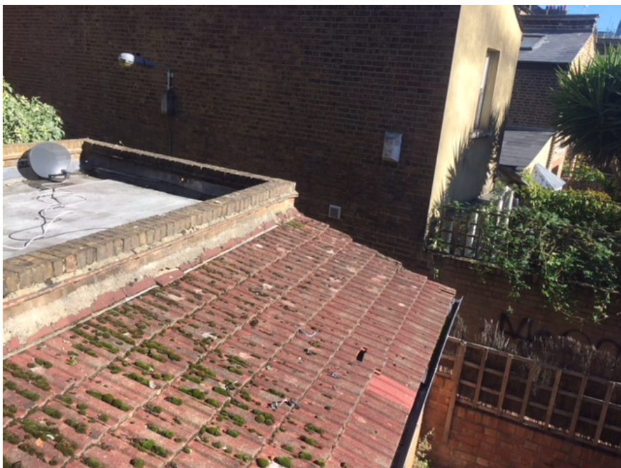
Photo 12 (above): Existing single storey rear extensions at No. 70 (flat roof) and No. 68 (pitched tiled roof) Highgate Road
