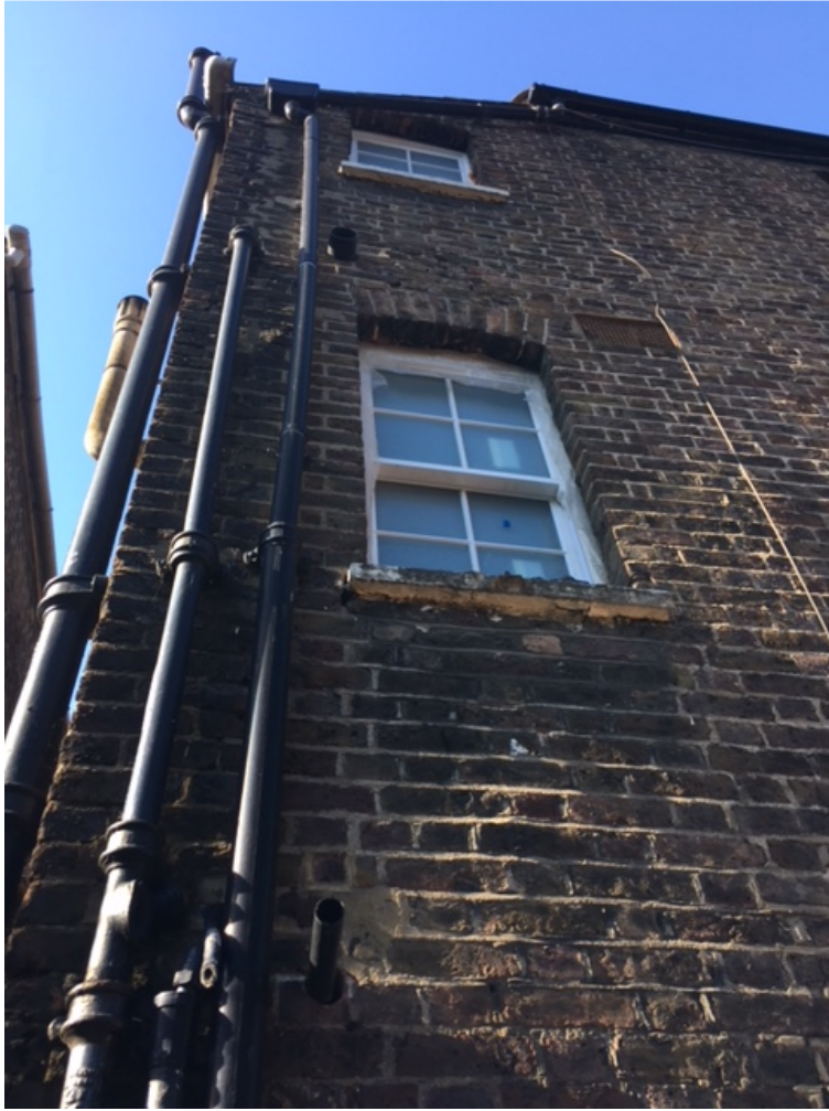
Photo 4 (above): Rear elevation of No. 68 Highgate Road, as-built first and second floor windows in situ
