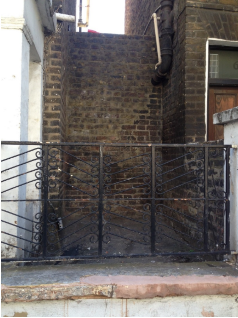
Photo 3 (above): As-built alterations to front elevation of pre-existing side extension
