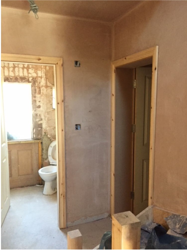
Photo 14 (above): As-built internal partition to ground floor WC, architraves and plastering. Partition and plastering proposed to be retained, other elements to be replaced or altered
