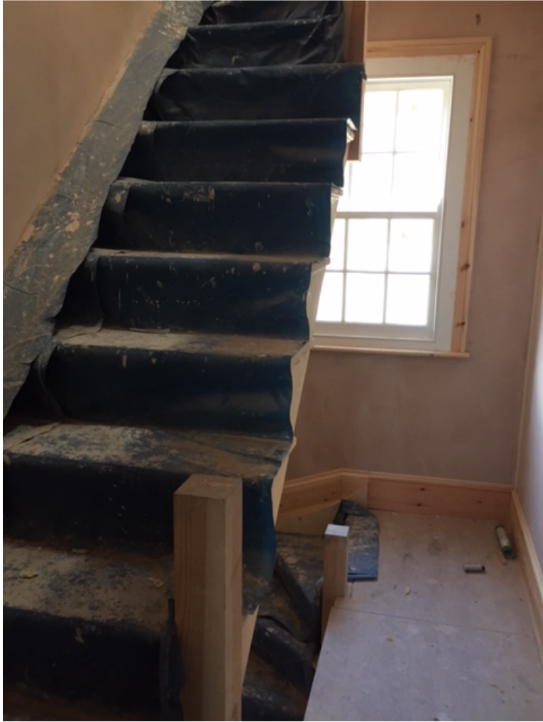
Photo 13 (above): As-built internal alterations to first floor landing including staircase, flooring, skirting boards, architraves and window. Plastering proposed to be retained, other elements to be replaced or altered
