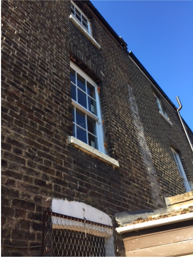
Photo 5 (above): Rear elevation of No. 68 Highgate Road, as-built first and second floor windows in situ
