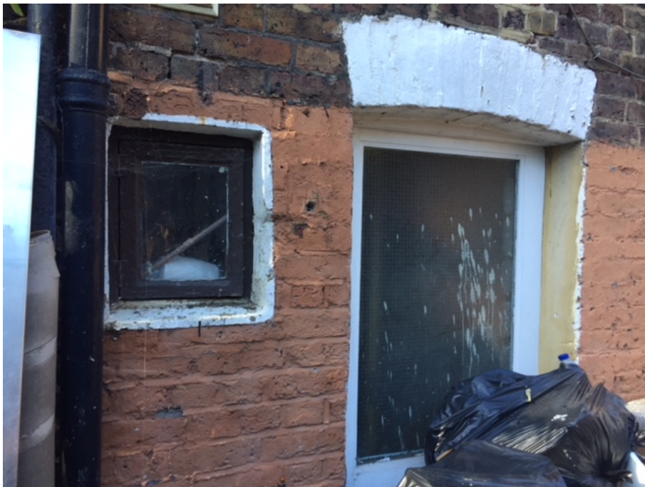
Photo 6 (above): View of existing ground floor rear window and door to be replaced
