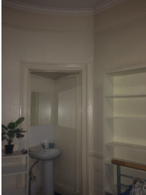
11. Front ground floor room at no. 110 – partial view of the curved wall, sink to be removed and wall to be made good to match existing; cornice to be repaired and retained.
