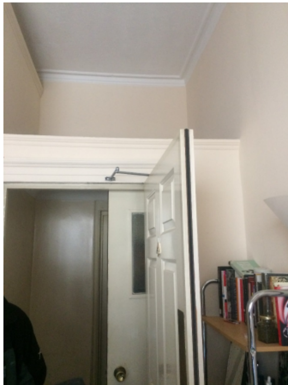
12. Existing partition walls to form entrance into rear room first floor at no. 109 – to be removed and plan form reinstated.
