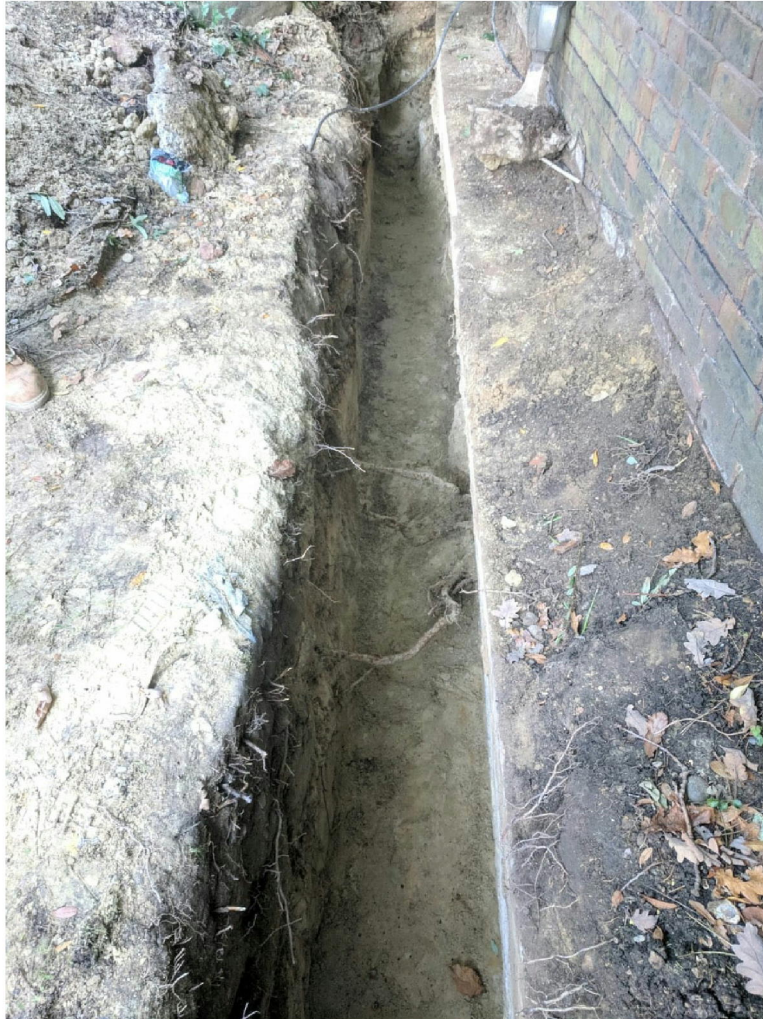
Photograph 1: No rooting from adjacent oak T1 within trial trench / beyond boundary wall foundations
