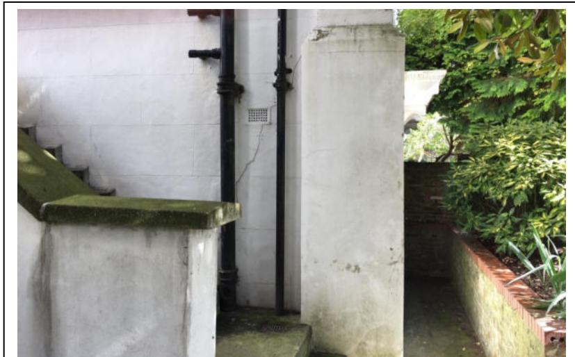
20. Cracking to front corner – 5 Agar Grove
