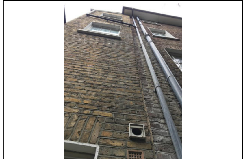
17. Rear elevation – 3 Agar Grove; note high level distortion up to side extension
