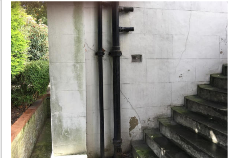
16. Cracking to front corner – 3 Agar Grove
