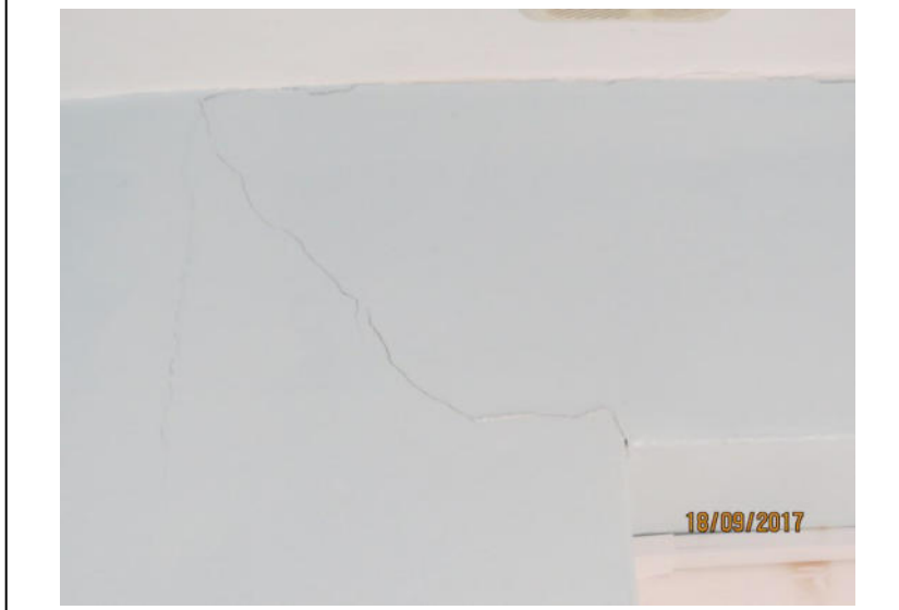
24. Crack to staircase side extension – 5 Agar Grove
