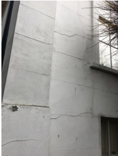
4. Cracking to stucco to front - 1 Agar Grove
