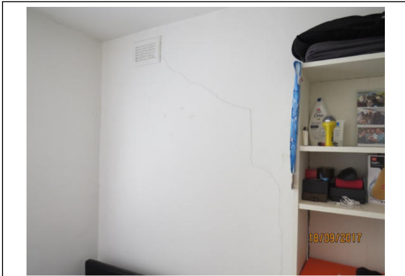
22. Internal crack to lower ground floor; mirrored by photo 20 – 5 Agar Grove
