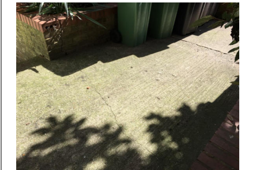
28. Cracking to concrete pathway – 1 Agar Grove
