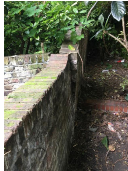
41. Cracked and displaced garden wall to rear of 3 Agar Grove
