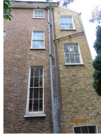
7. Rear elevation – 1 Agar Grove; note high level distortion up to side extension
