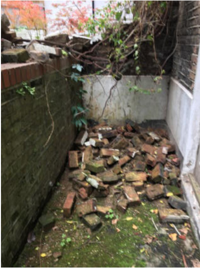
38. Collapsed garden wall to 5 Agar Grove with 7 Agar Grove
