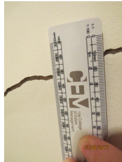
9. Close-up of crack in photo 8
