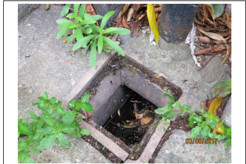
31. Blocked surface water gully – 1 Agar Grove
