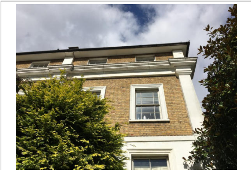
14. Front elevation; note crack over left hand window – 3 Agar Grove
