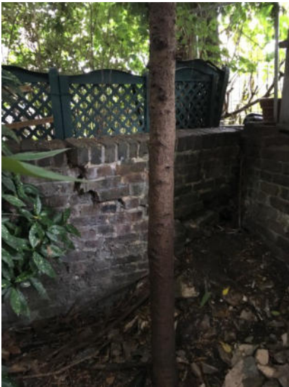
40. Cracked and displaced garden wall to rear of 5 Agar Grove
