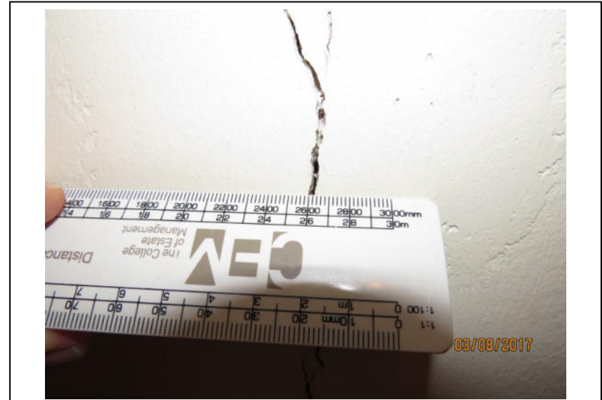
11. Close-up of crack in photo 10
