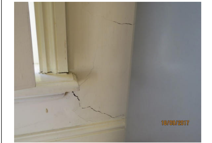
12. Internal crack to upper ground floor front wall – 1 Agar Grove
