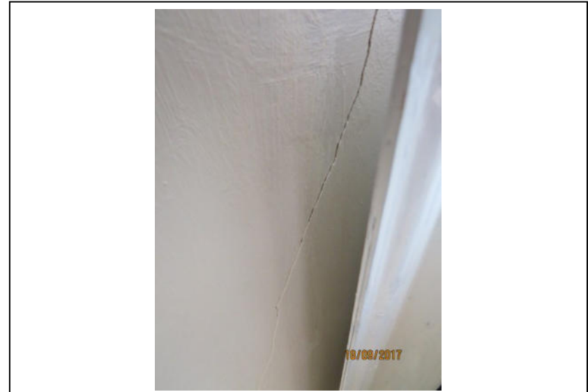
23. Internal crack to first floor front wall – 5 Agar Grove
