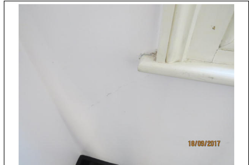
13. Crack to staircase side extension – 1 Agar Grove
