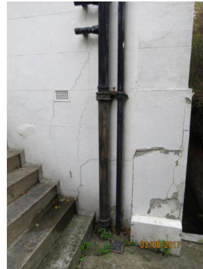
5. Cracking to front corner – 1 Agar Grove
