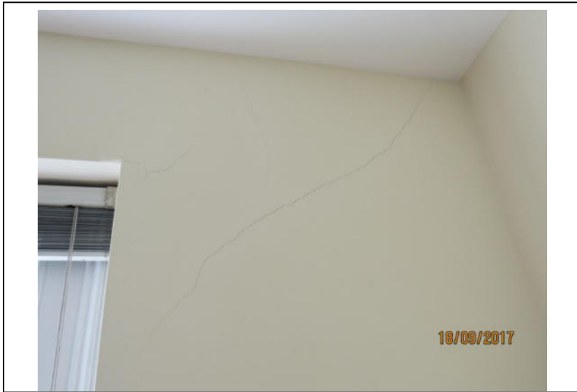
18. Internal crack to second floor front wall – 3 Agar Grove
