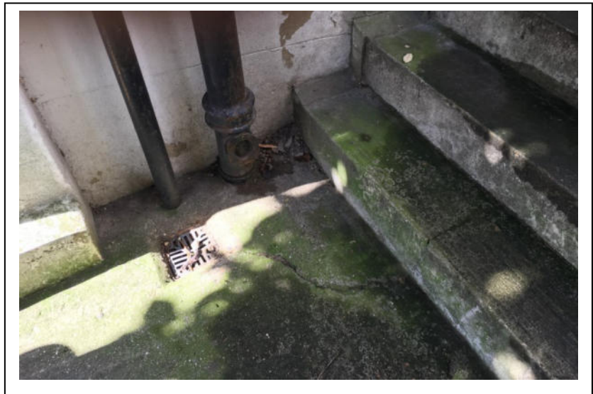
29. Surface water gully – 3 Agar Grove
