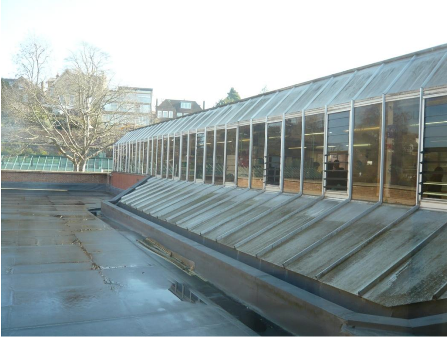
Fig.12 View from roof of 2010 addition to Sixth Form Centre – 1970s curtain walling to right
