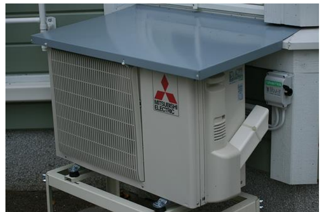
Figure 7: Outdoor unit of an ASHP
