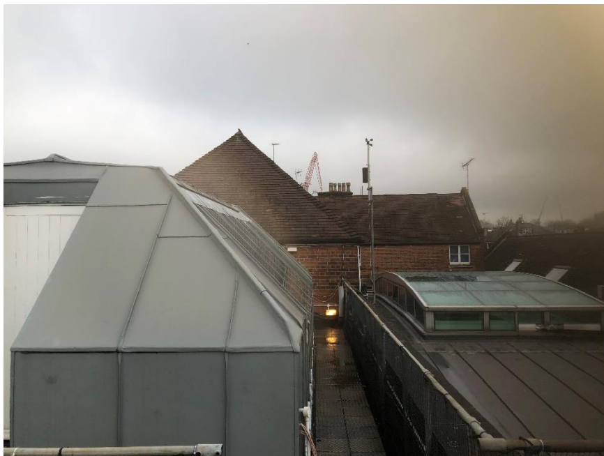
Photo 2. Roof of Building 1c with 'beehive' office visible in foreground and roof of Building 1a visible in background.
