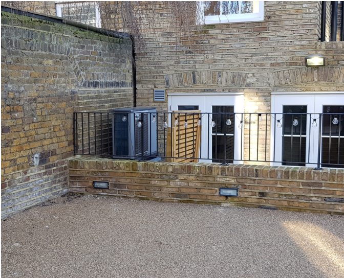
Air conditioning units installed to Princess Road in 2019, to a domestic property
