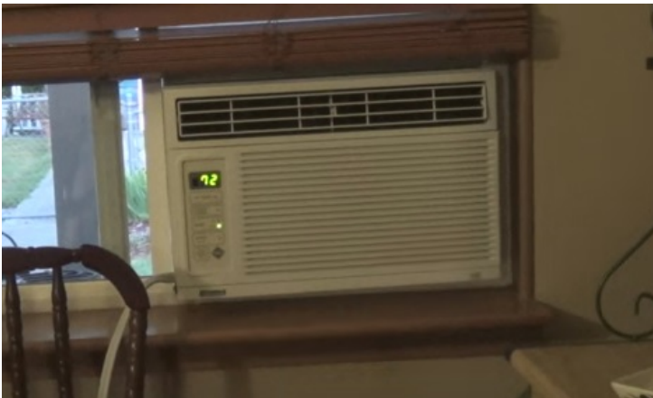
A window mounted air conditioning unit. These units are not energy efficient or environmentally friendly. We propose to cease use of these type of units with this application.
