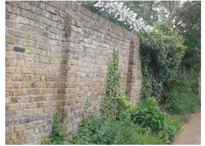
03 Existing brick wall to north side of private drive, south side of 29/33 Arkwright Road rear gardens.
