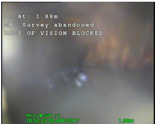
, 00:02:48, 1.88m Survey abandoned LOSS OF VISION BLOCKED
