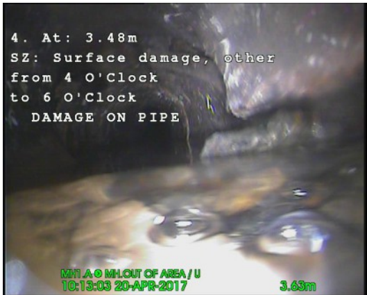
, 00:00:30, 3.75m Surface damage, other from 4 O'Clock to 6 O'Clock DAMAGE ON PIPE
