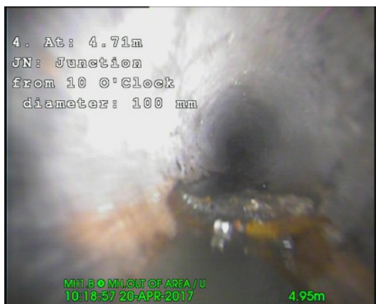
, 00:00:30, 4.98m Junction from 10 O'Clock diameter: 100 mm
