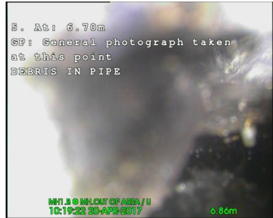
, 00:00:37, 6.88m General photograph taken at this point DEBRIS IN PIPE
