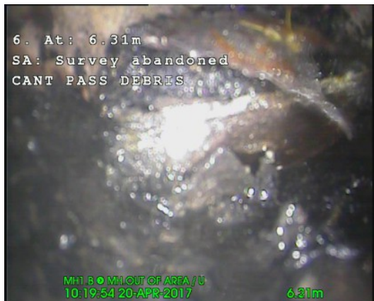
, 00:00:52, 6.19m Survey abandoned CANT PASS DEBRIS
