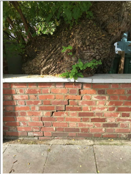
Image 1: taken from west and showing wall cracking and displacement.
