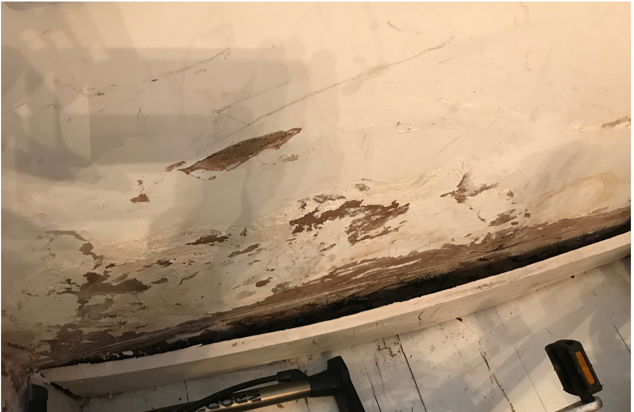
Damp damage in the cloakroom extends to the wall lining, floor finish and timberwork
