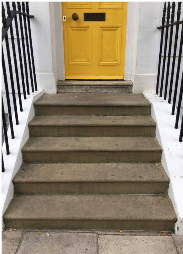
New proposed steps to raised ground floor to be clad in Portland stone to match neighbouring properties
