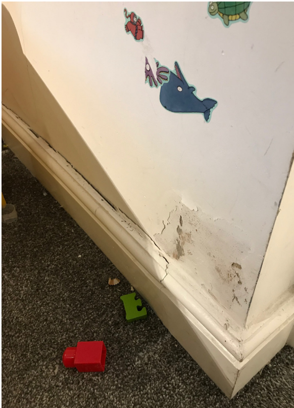
Existing damage to walls and timber-work in the front room onto the lightwell
