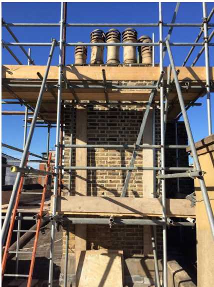
Fig 3 Existing chimney stack with scaffolding support to protect the chimney from collapse while application for repairs is underway.
