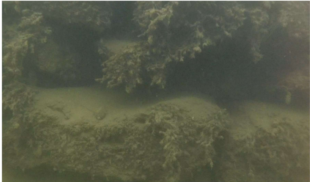
Figure 3.6: Identified large gap on the masonry blockwork wall
