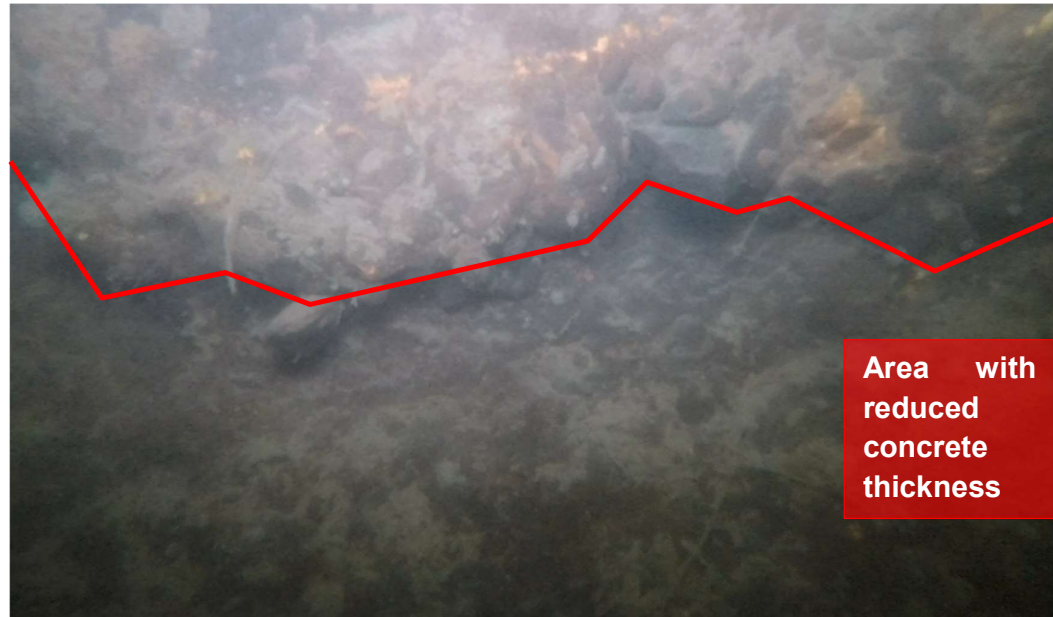
Figure 3.12: Photograph indicating a segment where the concrete layer is discontinued and its thickness is reduced.
