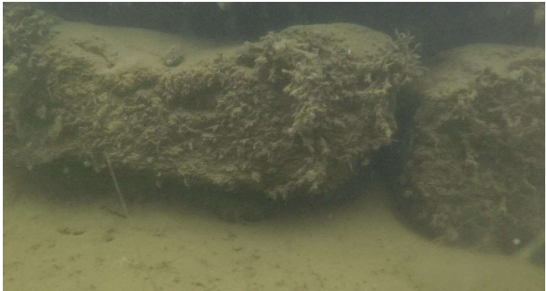
Figure 3.7: Scouring at the base of Section - 2 Masonry Blockwork Wall
