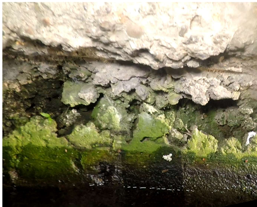
Figure 3.14: Photograph indicating the local damage of concrete extending above water level of Section 4
