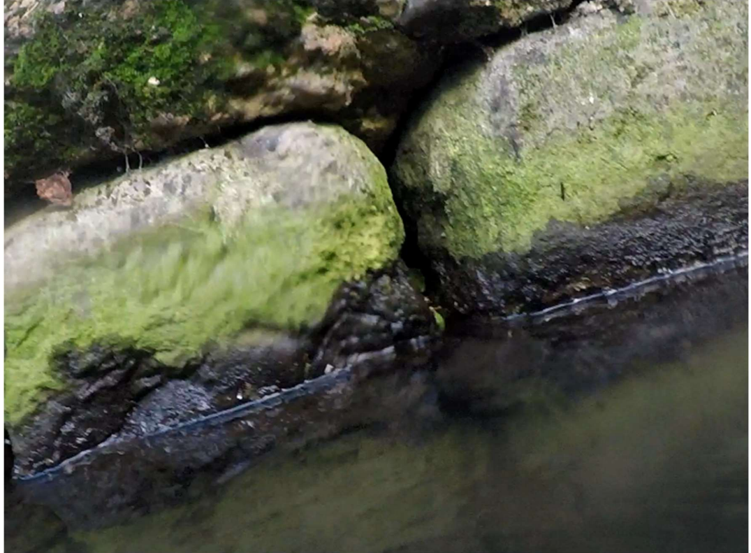
Figure 3.9: Formation of large gaps between masonry blockworks and concrete topping of Section 3
