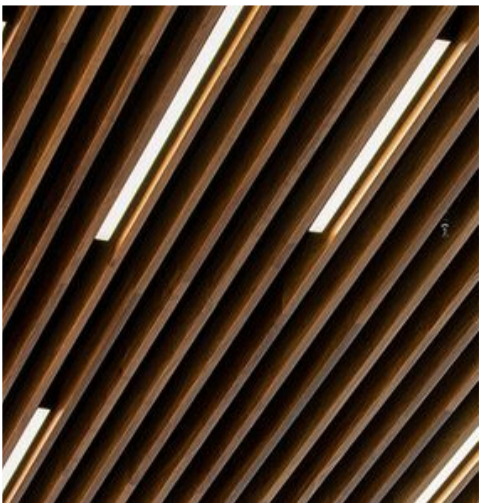
LED linears recessed within timber cladding
