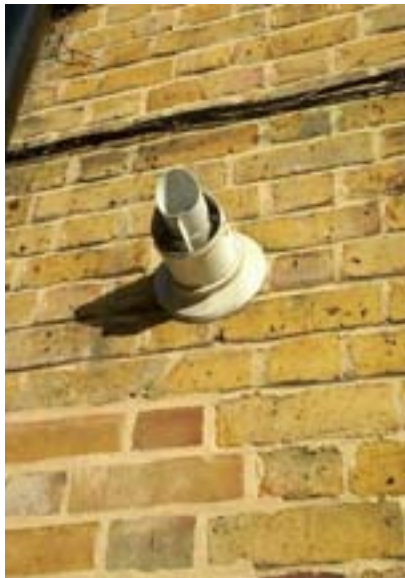
Image of installed boiler flue exit
