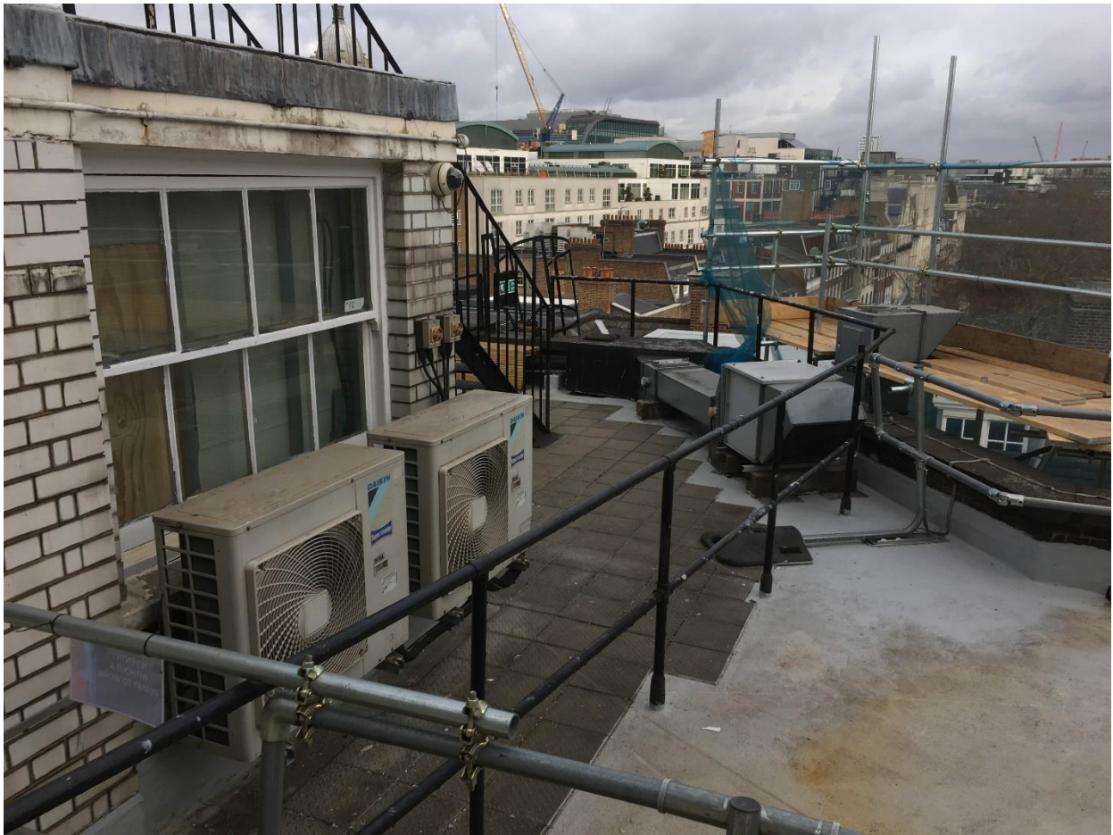
Figure 16. Existing AC units on the roof of the imperial buildings.
