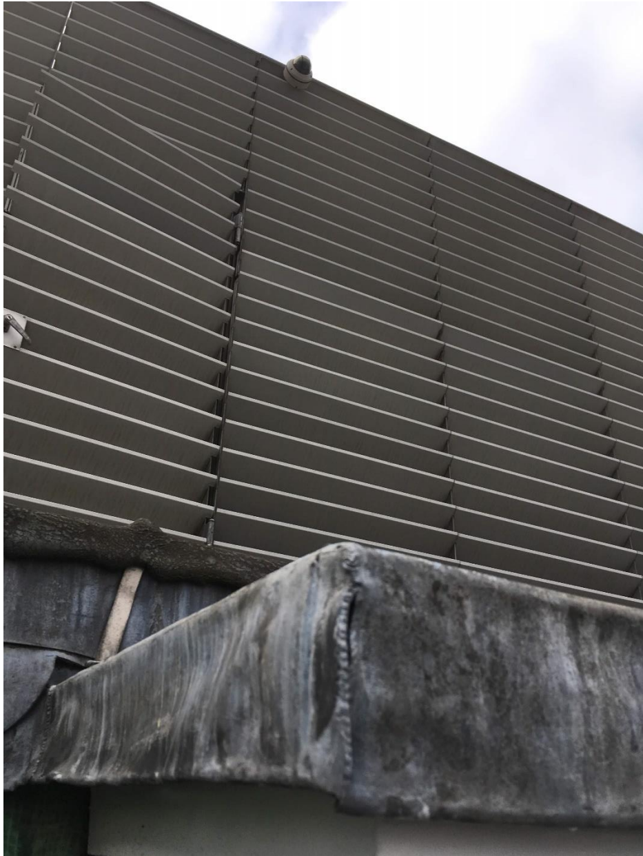
Figure 17. Detail view of existing screening to chiller units at roof level within the site.
