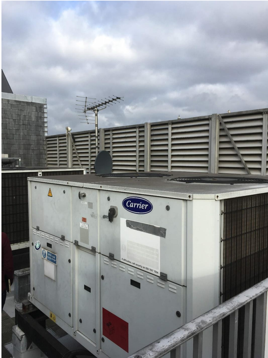
Figure 15. View of existing plant work to roof, note metal screen installed in the 1980s, preventing extensive views to and from the surroundings.
