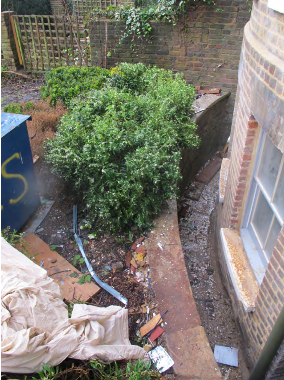
Fig. 4.3A Existing rear lightwell, unprotected edge
