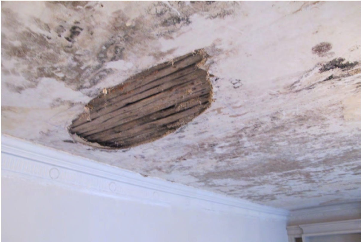
Fig. 2.2C Water damage and failing lime plaster ceiling
