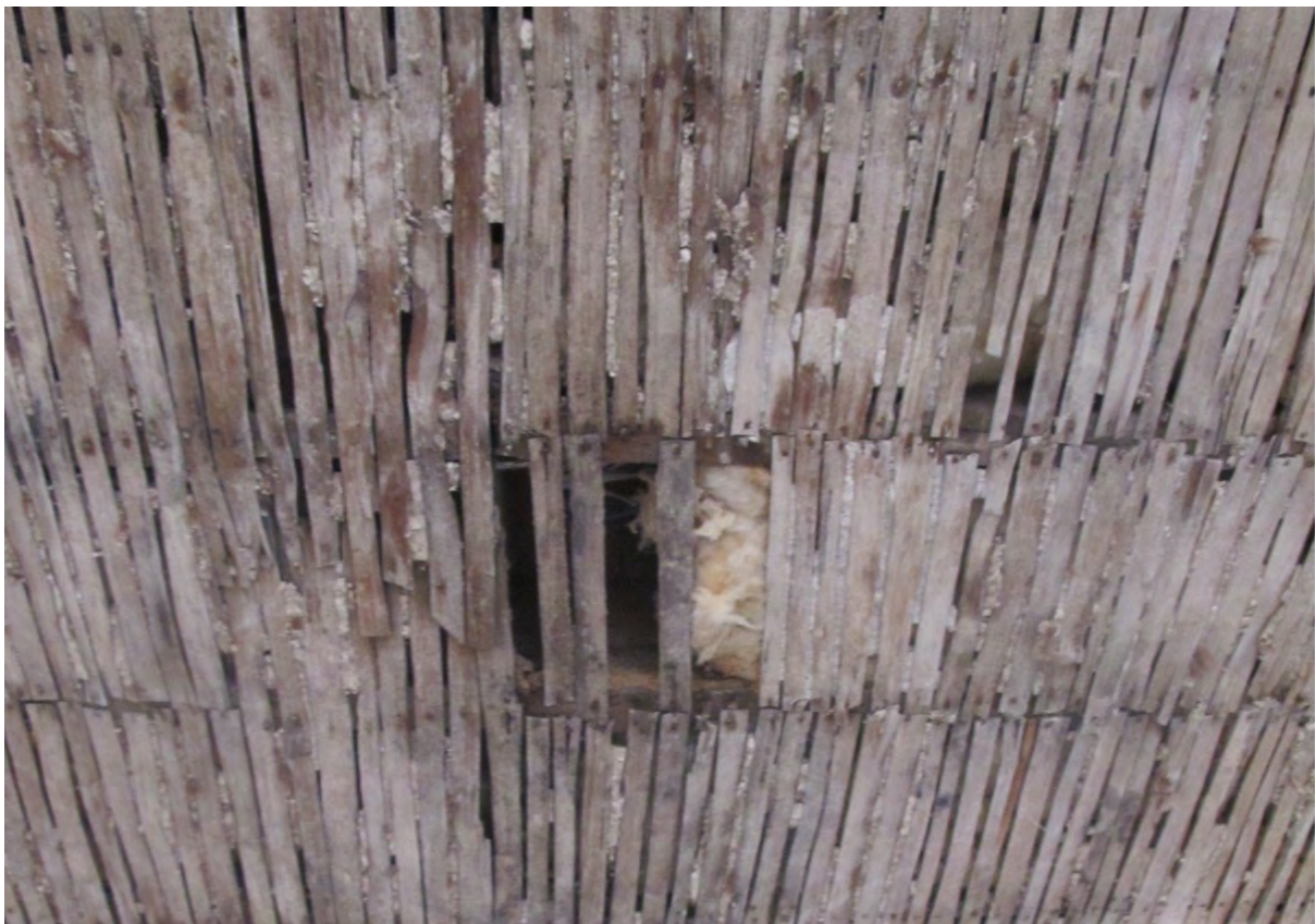
Fig. 2.2D Frail and water damaged lathing [Note laths also set tightly together]
