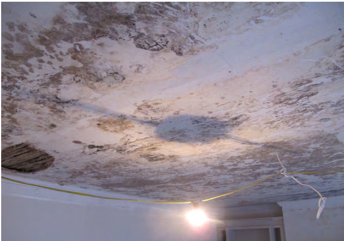
Fig. 2.2B Removal of over-boarding, revealing mould growth and water damage to original lime plaster and lath ceiling
