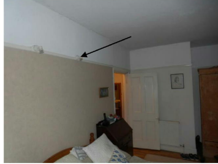
Basement flat 1 – unrelated damage
