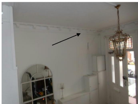
Communal hall – crack
