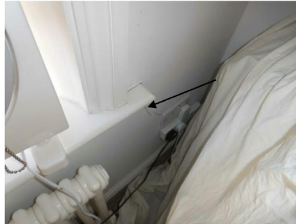
Flat 3 rear bedroom – unrelated damage
