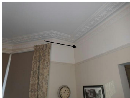
Flat 3 front lounge - crack
