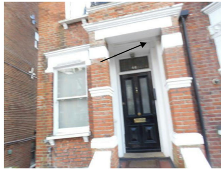
Cracks around front door
