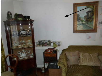
Flat 2 front lounge – crack
