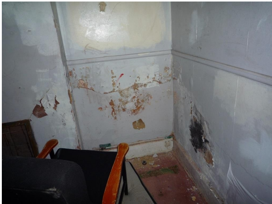
Picture 2 – House 1, Severe damp in ground floor living room
