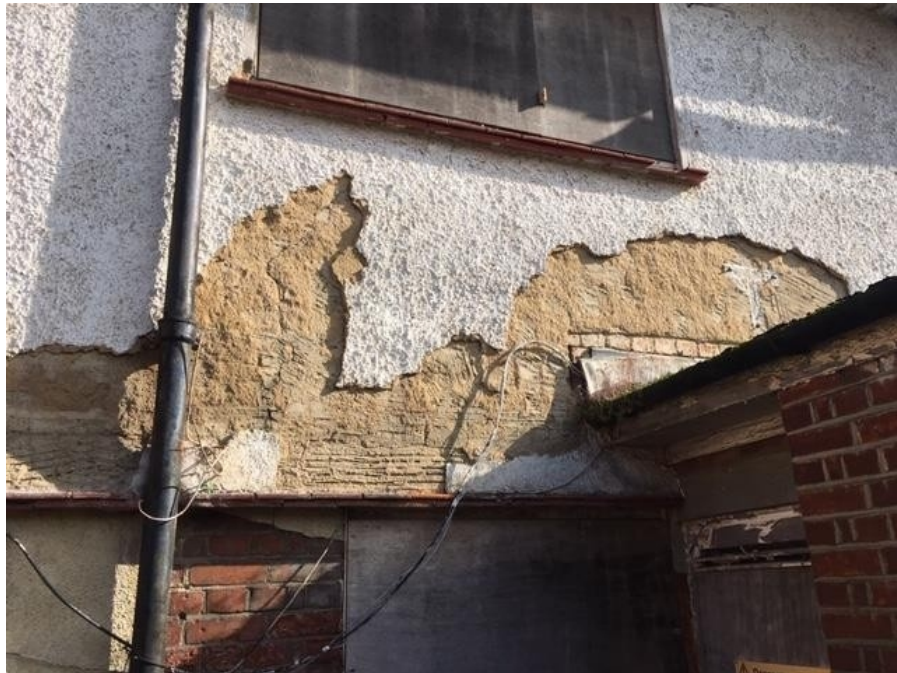
Picture 22 – House 2, main house rear elevation with large areas of original and render coming away.
