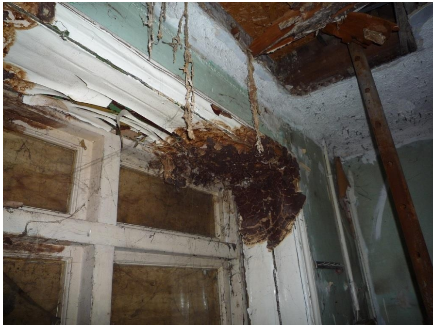
Picture 12 - House 4, Severe dry rot in window timber in kitchen
