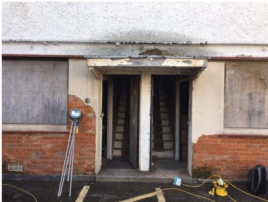
Picture 16 – Houses 1 & 2, front doorways and dilapidated timber porch
