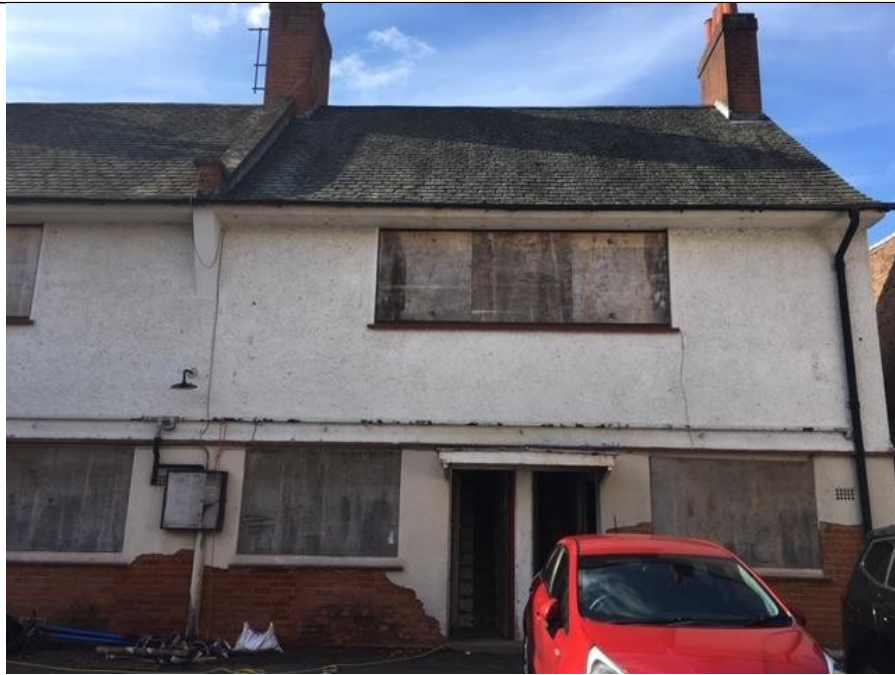
Picture 15 – Houses 3 & 4, front elevation with l/l render coming away
