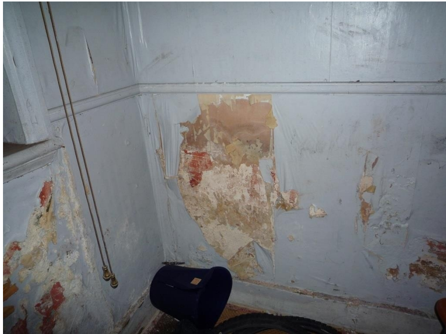
Picture 1 – House 1, Severe damp in ground floor living room
