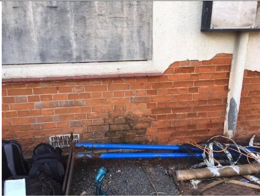
Picture 17 – House 2, low level brickwork face powdering and delaminating on front elevation where rendering has come away.
