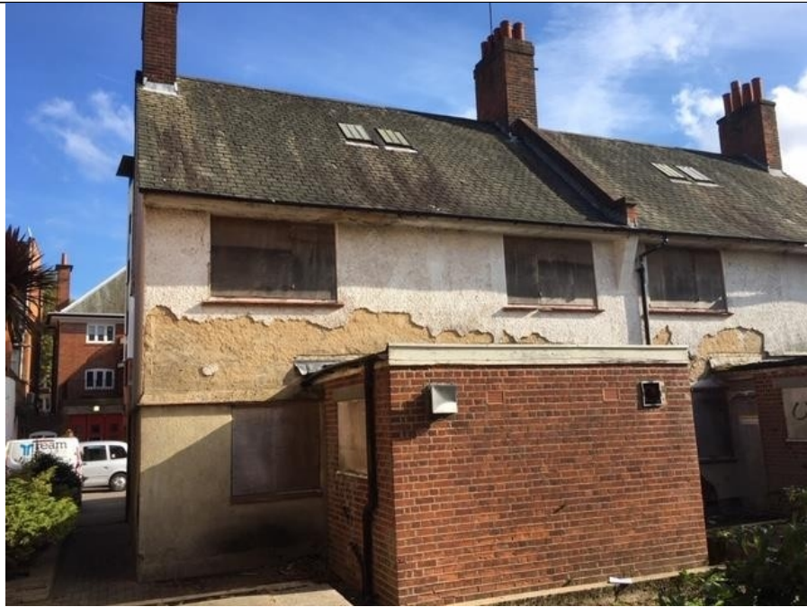
Picture 19 – Houses 3 & 4, rear addition and main house elevation with large areas of render coming away.
