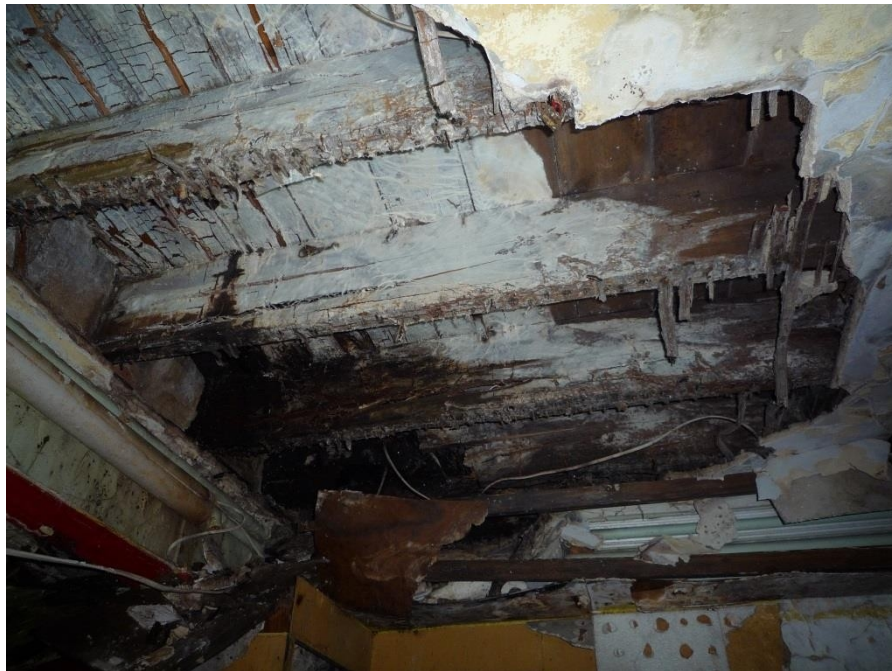
Picture 8 – House 2, Severe dry rot in timber floor over kitchen
