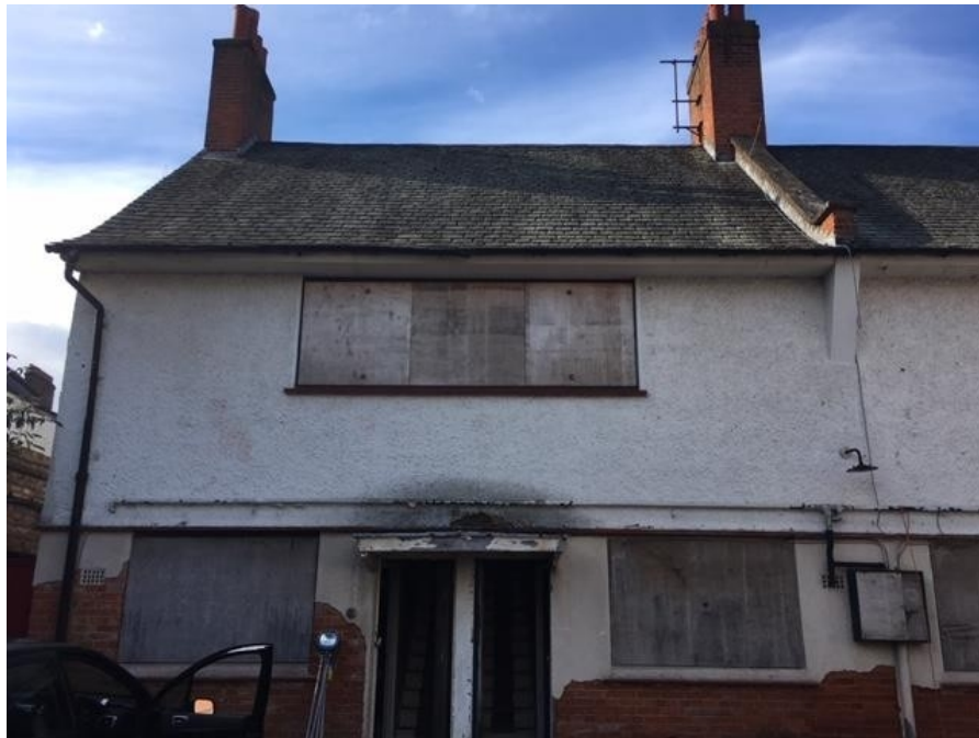
Picture 14 – Houses 1 & 2, front elevation with l/l render coming away
