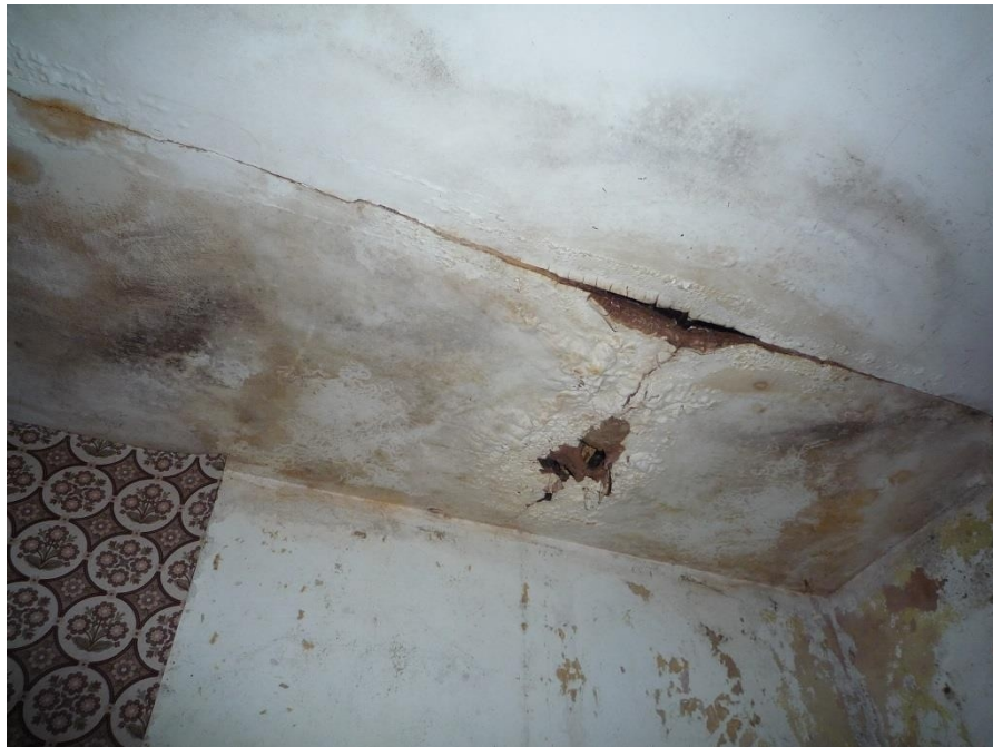
Picture 6 – House 2, Wet and probable joist rot in ceiling to rear addition
