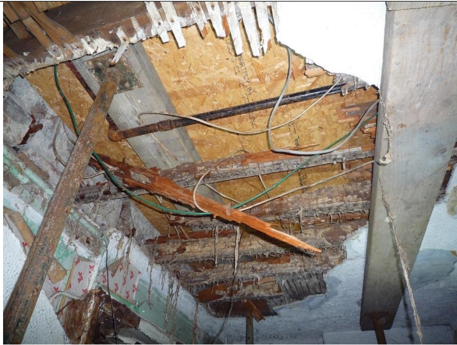
Picture 11 - House 4, Severe dry rot in timber floor over kitchen
