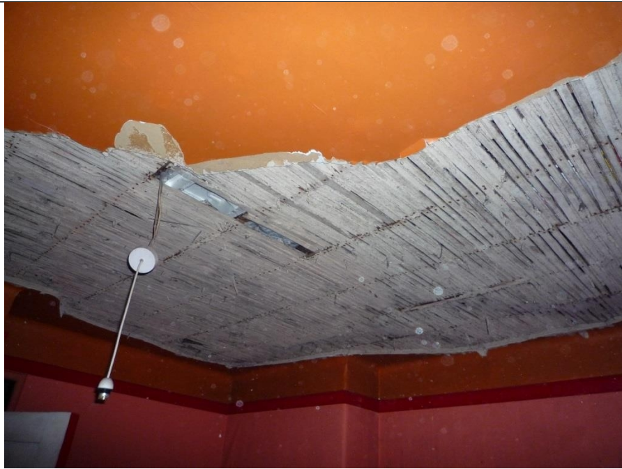
Picture 9 – House 2, Ceiling plaster down in bedroom 1
