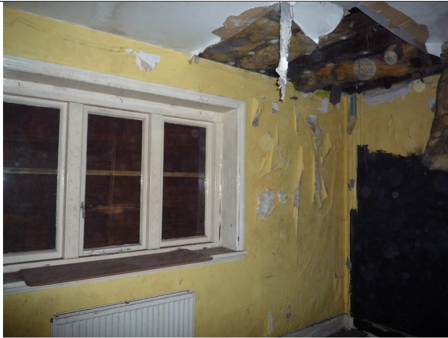
Picture 5 – House 1, Damp and ceiling plaster down in bedroom 2
