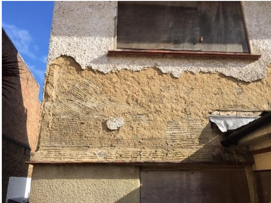
Picture 20 – House 4, main house rear elevation with large areas of original render coming away.
