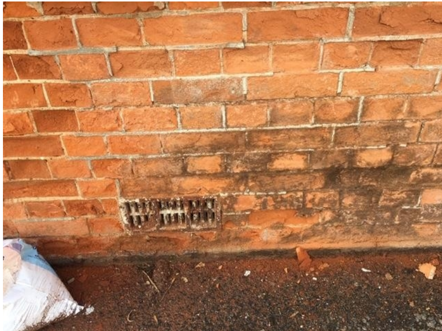
Picture 18 – House 3, low level brickwork face powdering and delaminating on front elevation where rendering has come away.
