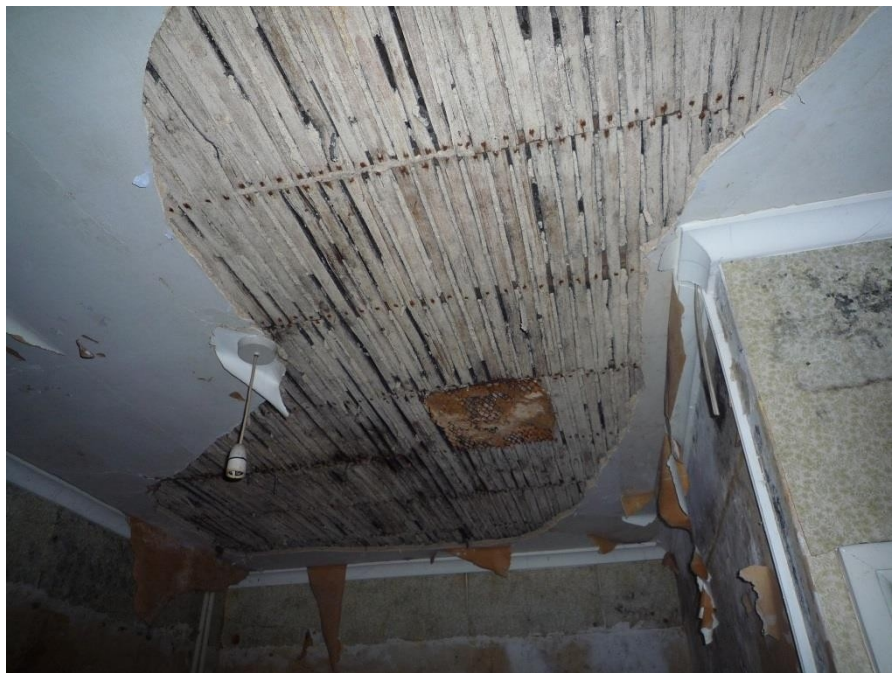
Picture 10 - House 3, Ceiling plaster down in bedroom 2
