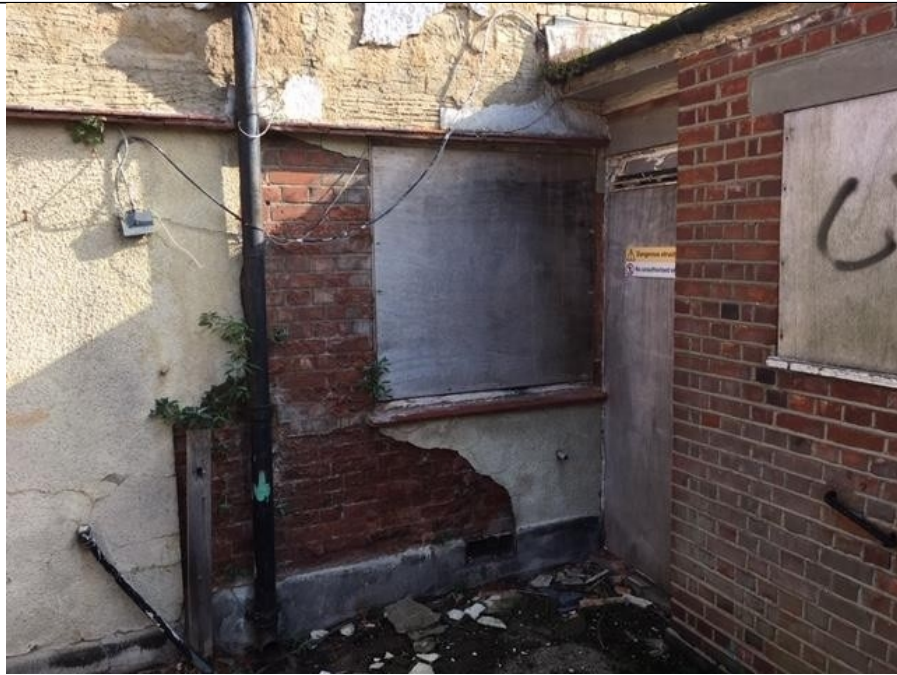
Picture 21 - House 2, main house rear elevation with large areas of original and newer render coming away.
