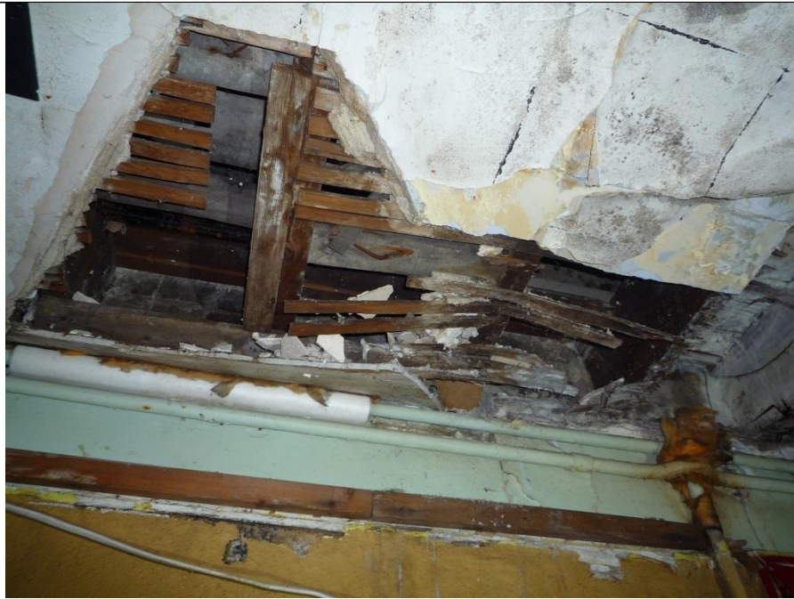
Picture 7 – House 2, Severe dry rot in timber floor over kitchen
