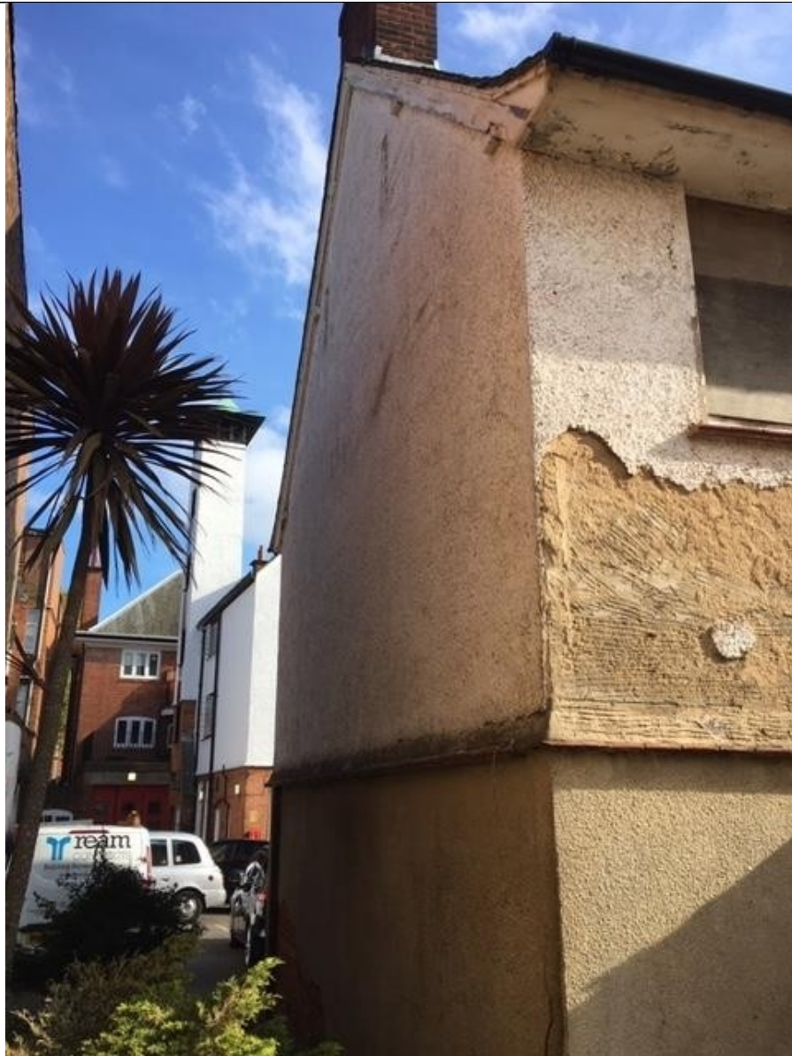
Picture 23 – House 4, Flank gable wall with loose and hollow rendering at low level and some missing render.
