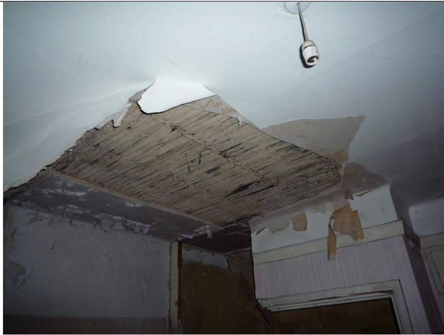
Picture 13 – House 4, Ceiling plaster down in bedroom 1, similar in living room
