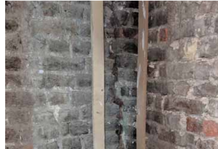
2 Front facade delamination
