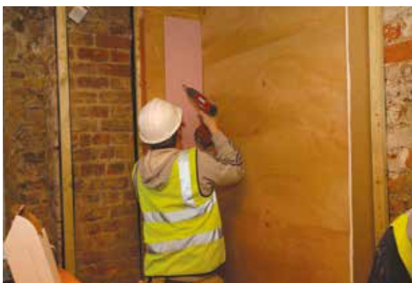
Plywood installed over insulation was used to take the weight of heavy fixtures and fittings in the kitchen.
