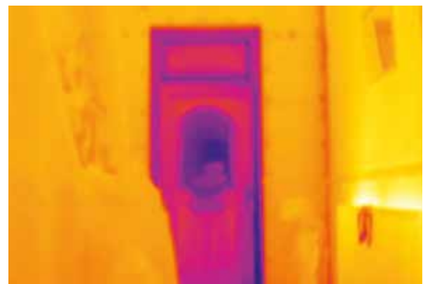
Thermal Image of External Gable Wall after IWI (Outdoor Ambient Air Temperature = 0.0°C & Wall Surface temperature Defined in Area AR01 = 0.8°C).
