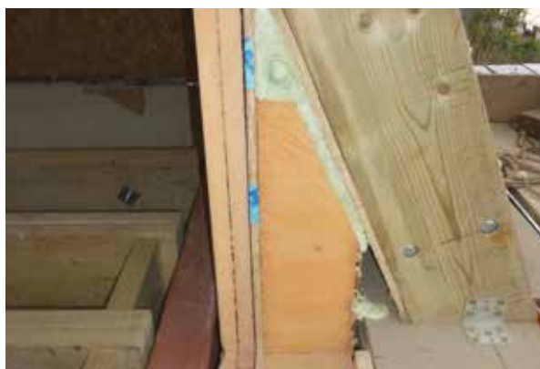
Detail showing the wall construction with the OSB airtightness layer and steel used to re-hang the floors.
