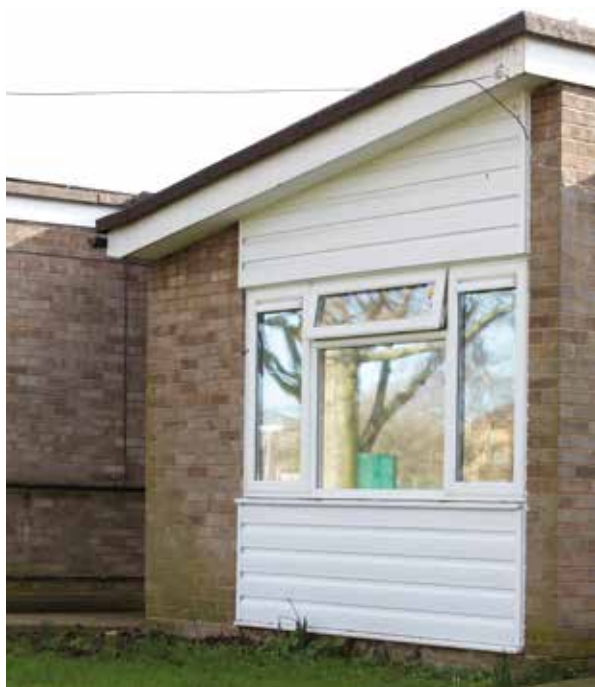
Ten under-insulated bungalows were funded as part of the £1.2 million ReallySmartHouse project.
