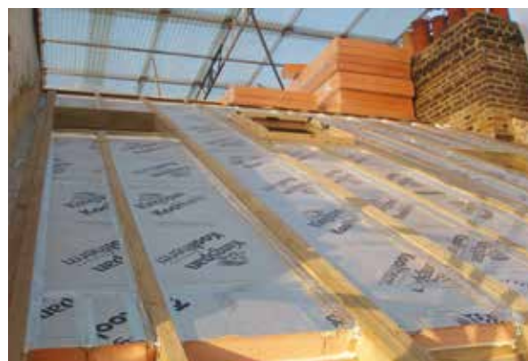
Careful taping and sealing of joints with Kingspan Kooltherm ® K7 Pitched Roof Board.
