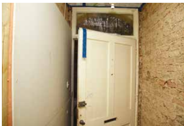
Kingspan Kooltherm ® K18 Insulated Plasterboard used in the hallway encroached as little as possible on available space.
