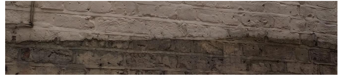
EXISTING AGED BRICKWORK (7 Anglers Lane)
