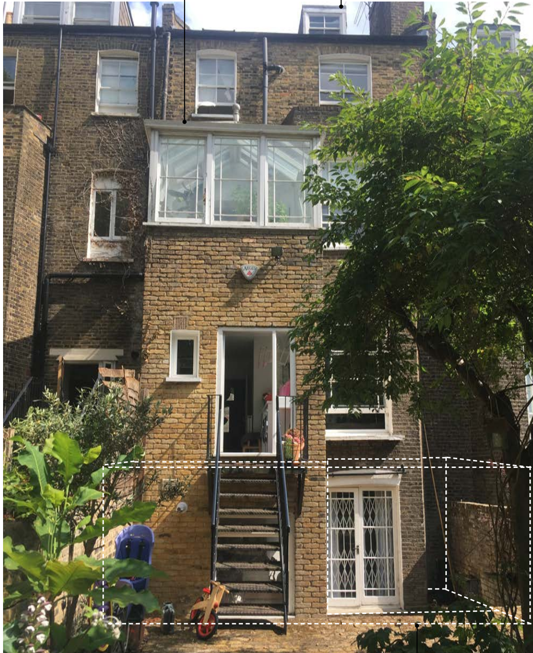
View of 81 St Augustine's Road garden elevation. Extent of the works indicated.
