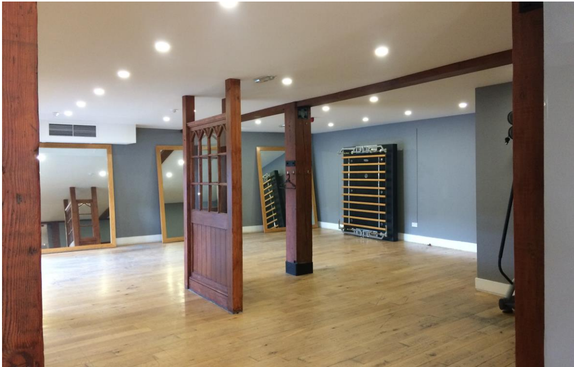
Figure 2: Ground floor with original timber posts and timber and glazed screens in non-original position.
