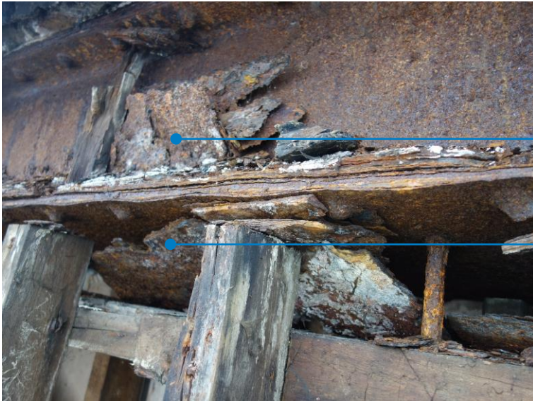
1.3 Delamination of existing steel truss top chord.
