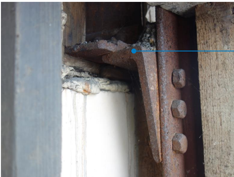
1.5 The connection of the existing roof beam to the truss vertical was observed below the brick parapet.
