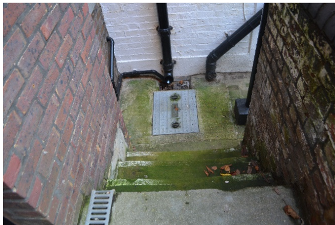
Manhole to be connected into in front of the rear wall where new window is proposed.
