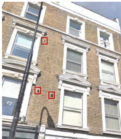
fig. 2: Front flue terminals at first and second floor levels at nos. 4 & 6 England's Lane
