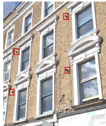
fig. 3: Front flue terminals at first and second floor levels at nos. 22 & 24 England's Lane
