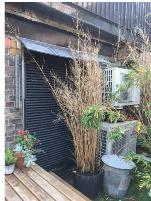
3.2.22 Existing services to rear terrace
