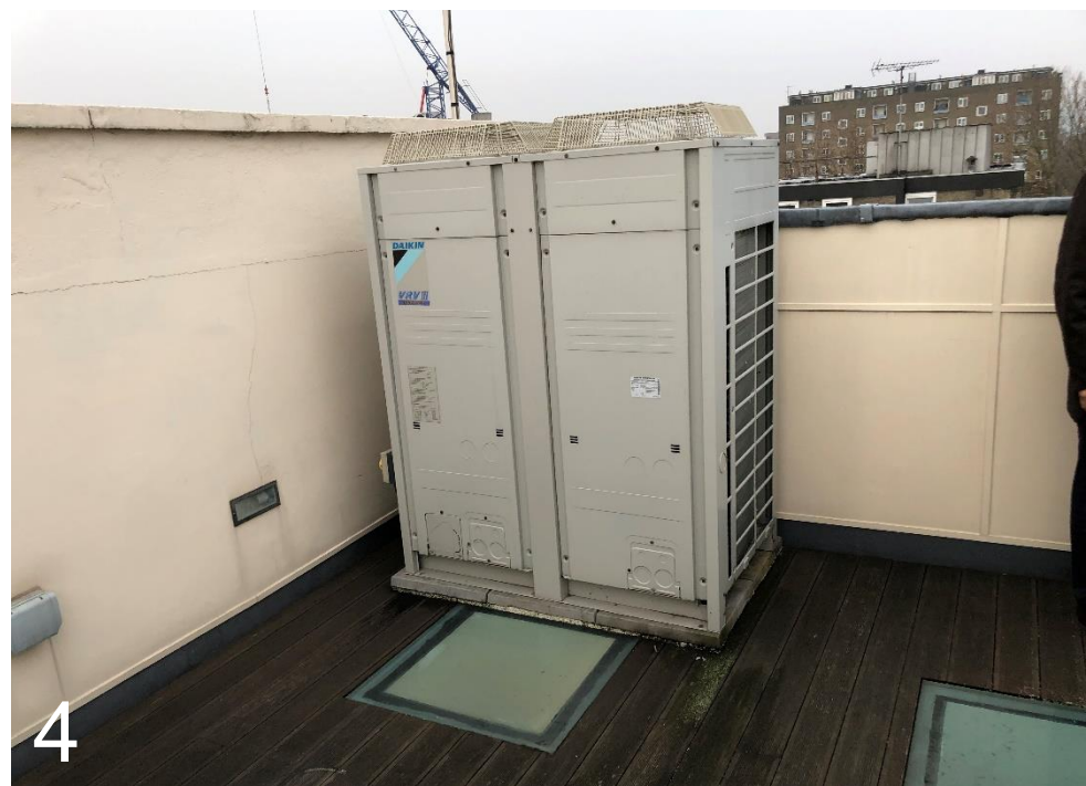
4 Existing air conditioning unit on raised level of Roof Terrace
