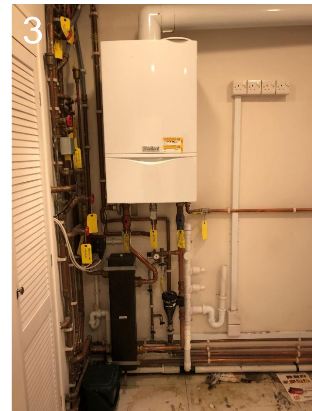
3 Existing boiler in Utility room, opposite sink
