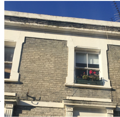
Rendered surround to new ground floor windows to match second floor windows
