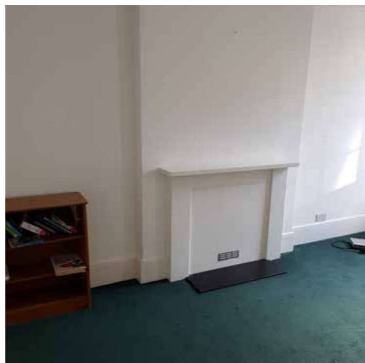
14 - Covered fire and later addition surround
