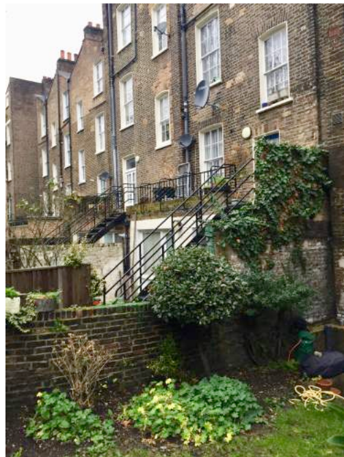
No. 15 & 17: Black metal access stairs from rear terraces to gardens (view from garden of No. 11)
