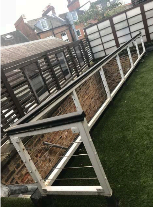
Photo 4 - View from the opposite side of the Terrace looking at the metal balustrade and timber screens.
