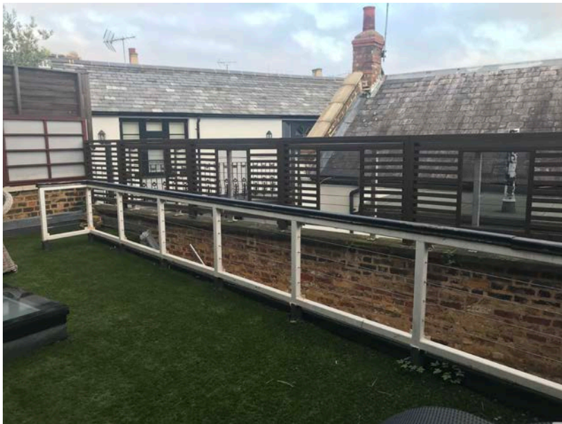
Photo 3 - View from the Terrace looking at the metal balustrade and timber screens.
